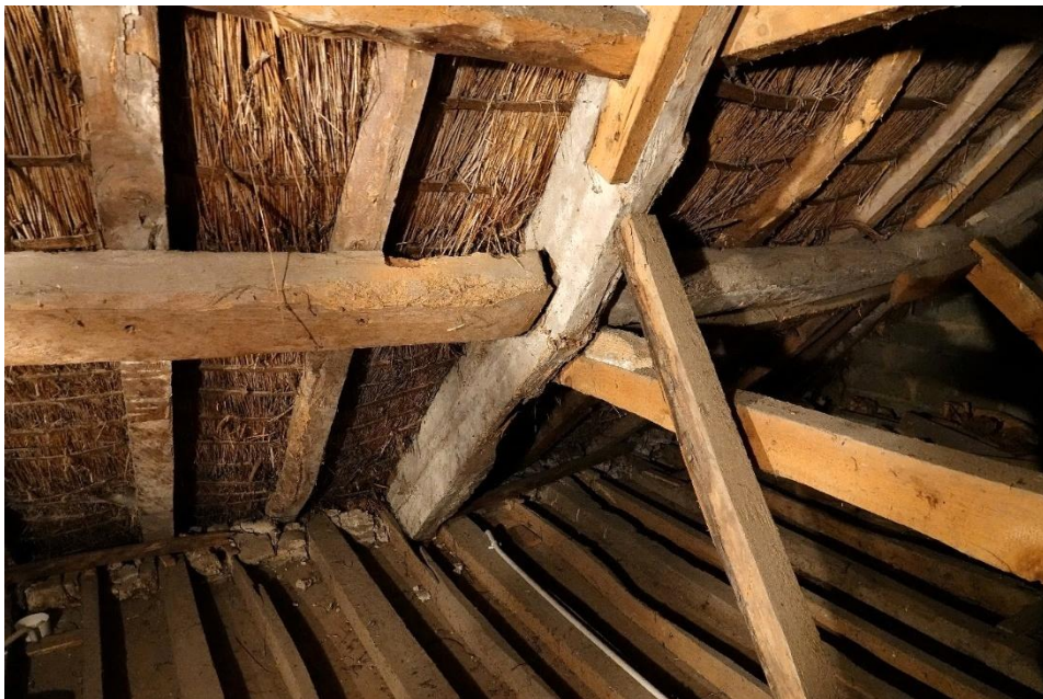
Fig.88 – Truss T2, the failed NW principal. Note the absence of a tiebeam
