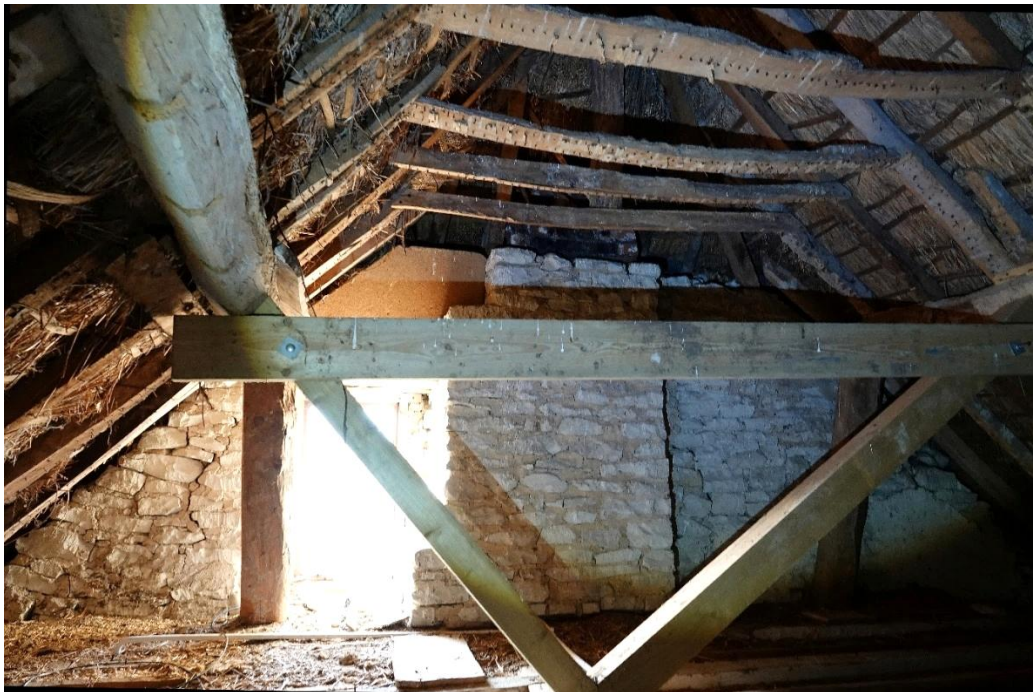
Fig.64 – General view of the SW end bay, looking to the gable window and stack – note the nails from lost laths
