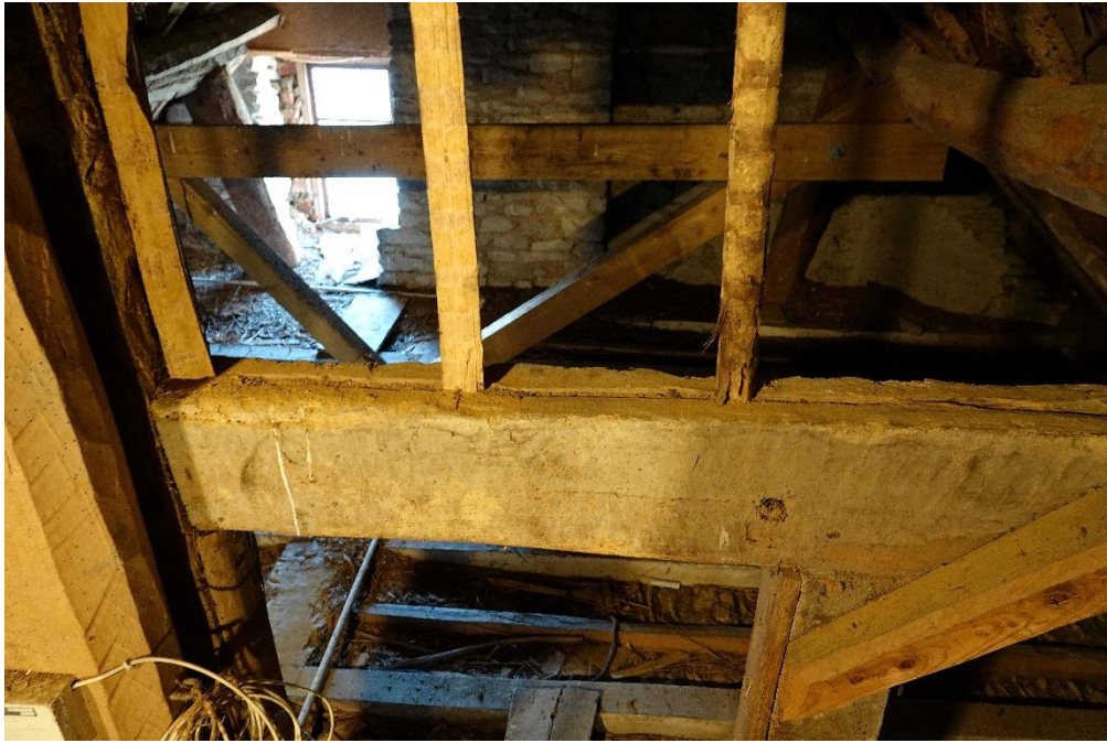
Fig.77- details of truss T1 showing the stave groove in collar upper face
