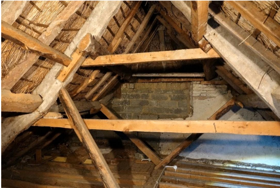
Fig.87 – Truss T2, looking NE to the end wall. On the left, the principal has failed and is now propped extensively. This view also shows the blockwork in the end wall
