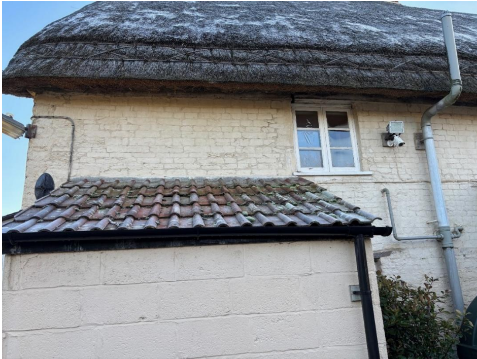
Fig.29 Detail of coursed rubble of rear elevation, and disturbed stonework to left window jamb
