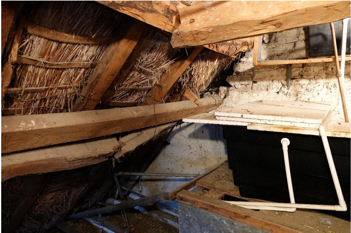
Figs.78 & 79 - the bay NE of T1 – (above) the front slope, showing failed butt purlin (below) the rear slope, again with a failed purlin and above that, an added upper purlin held by a spacer beam, birdsmouthed and nailed
