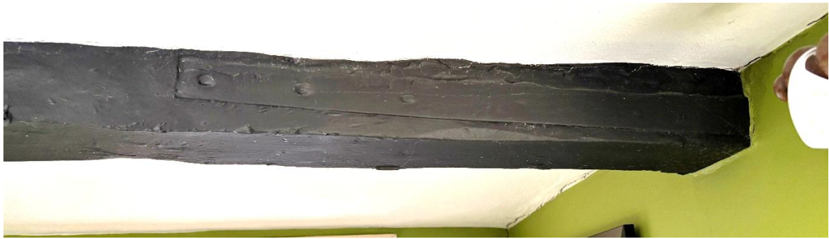
Fig.55 West face of east transverse beam between stack and front wall with 20 th century metal strapping
