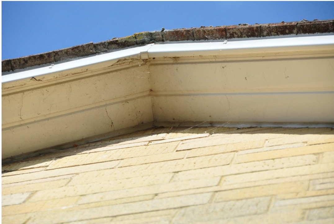
Plate 5 gable end well sealed negligible potential for birds or bats
