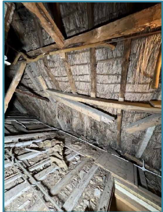
West Cell - Failed Purlin
