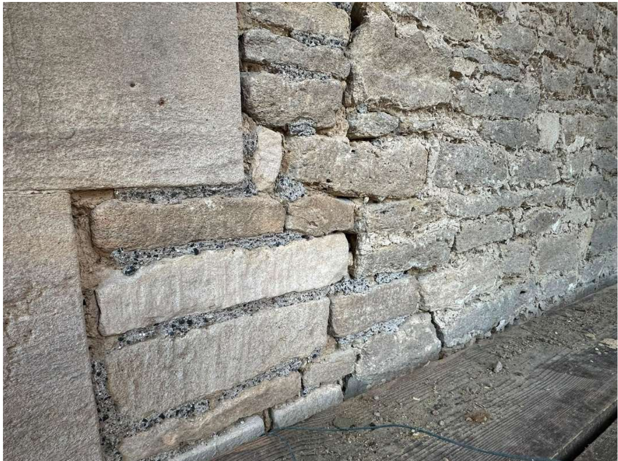
Fig 4: Group of Photos: Rubble stone with open mortar joints and cement repairs
