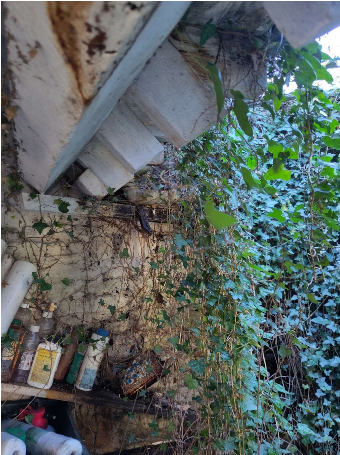
Fig 11: Dilapidated wood store interior
