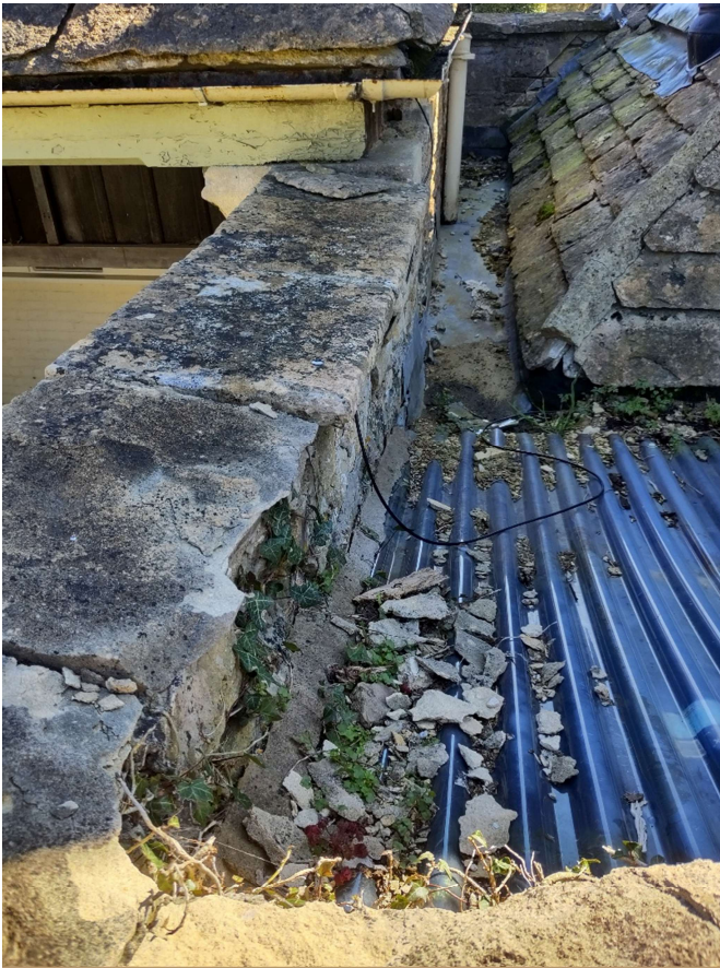
Fig 10: Weathered stone parapet to be replaced
