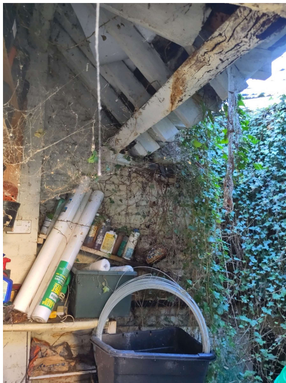
Fig 9: Internal wood store – rotten rafters and vegetation
