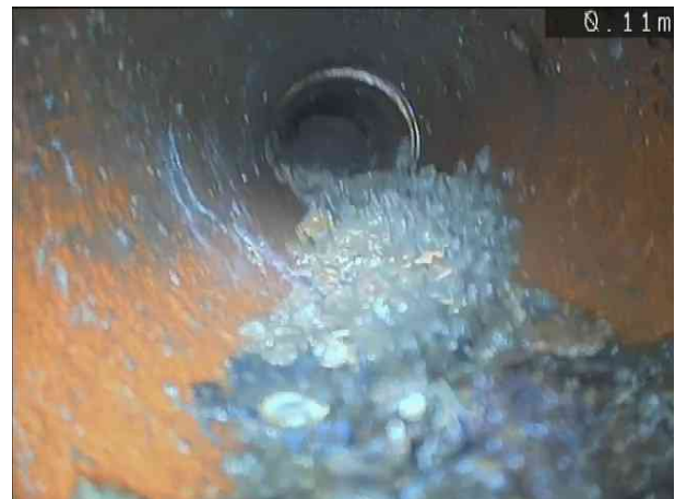
UnknownX_aa392f14-f072-4e23-8d57-0af68de4823c_20241106_122454_667.jpg, 00:00:14, 0.11 m Settled deposits, fine, 15% cross-sectional area loss, start
