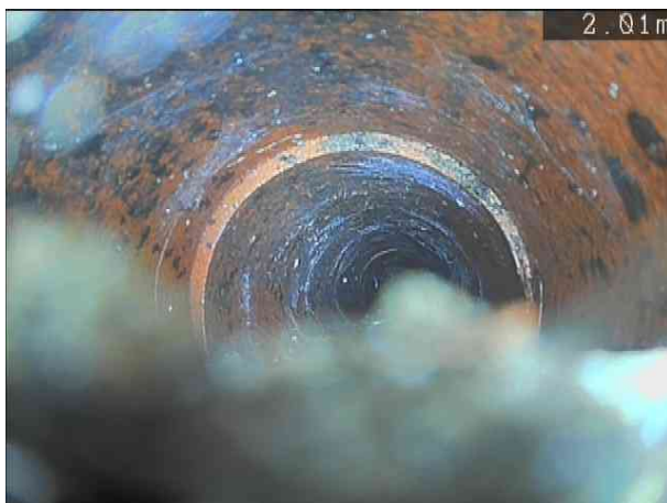
RWWG1X_ebeea0d1-1a22-453a-8d32-a98129a4e5da_20241106_122040_552.jpg, 00:00:49, 2.01 m Crack, circumferential from 4 o'clock to 11 o'clock
