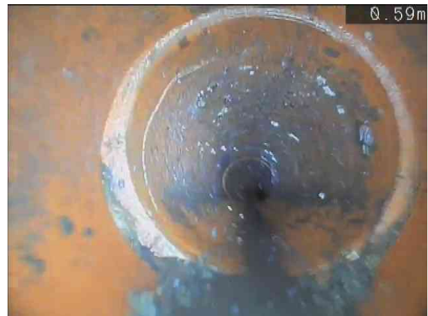
MH2X_493d89ce-f528-4eec-a012-1d1f96db270c_20241106_123134_672.jpg, 00:00:16, 0.59 m Crack, circumferential from 8 o'clock to 12 o'clock
