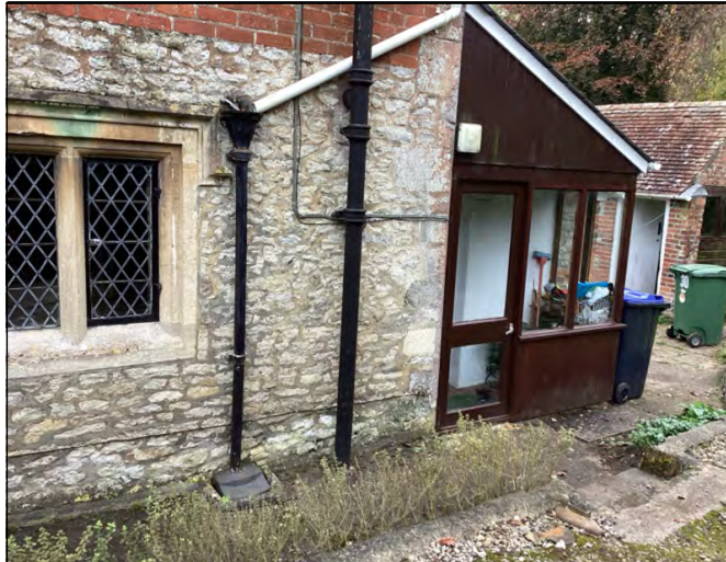
rain water cross connection at RWWG1
