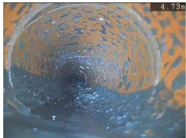
MH2X_1b3c6750-1a7d-4961-8f1c-dcd46c15ad4a_20241106_123351_921.jpg, 00:00:35, 4.73 m Crack, circumferential from 10 o'clock to 5 o'clock
