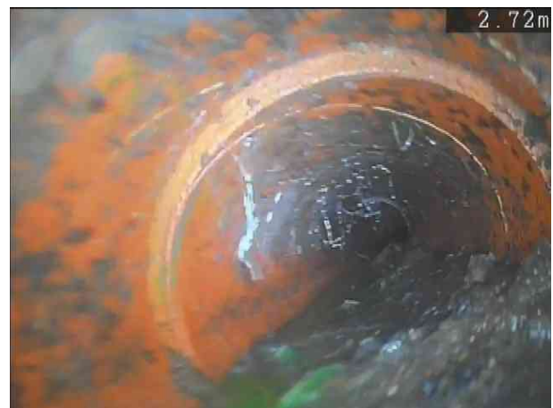
RWWG1X_86e6af7c-43b0-4f40-9652-0ae3e08a8b3b_20241106_122100_357.jpg, 00:00:56, 2.72 m Cracks, spiral from 9 o'clock to 5 o'clock
