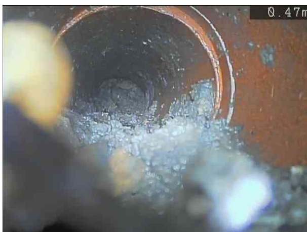
UnknownX_a8f858ec-b9ad-4292-a37d-4d0c5fb1dbe1_20241106_122508_704.jpg, 00:00:17, 0.47 m Fracture, circumferential from 12 o'clock to 4 o'clock
