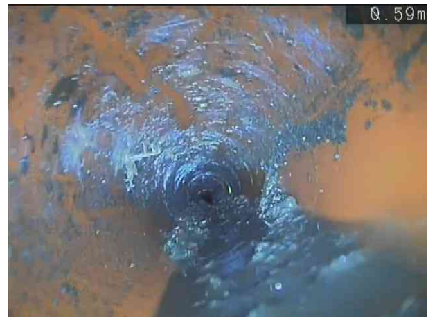
MH1X_e0a5b025-1650-4098-ba8a-69178dd9b2d3_20241106_122746_902.jpg, 00:00:14, 0.59 m Settled deposits, fine, 15% cross-sectional area loss, start
