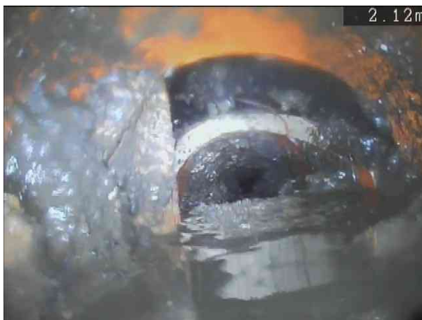
MH1X_147ddf87-d27d-45c7-b92f-d7a50c0d1b6e_20241106_122857_182.jpg, 00:01:00, 2.12 m Broken pipe from 9 o'clock to 3 o'clock
