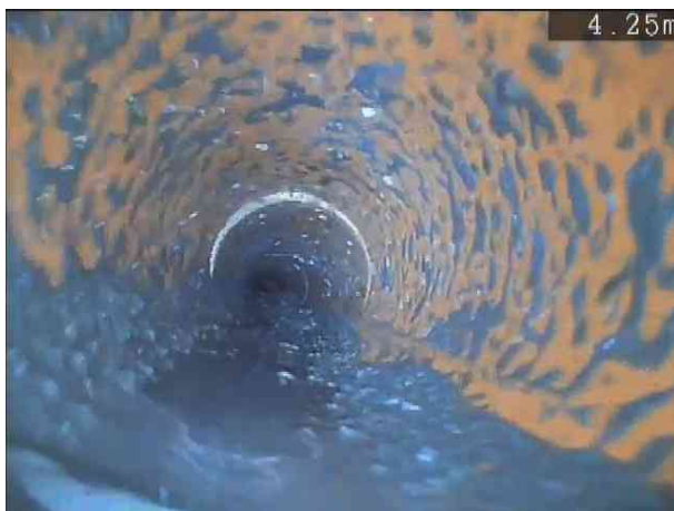
MH2X_8dca36d0-ac9d-4d5f-a4de-f5b96a658363_20241106_123248_012.jpg, 00:00:34, 4.25 m Settled deposits, fine, 15% cross-sectional area loss, start
