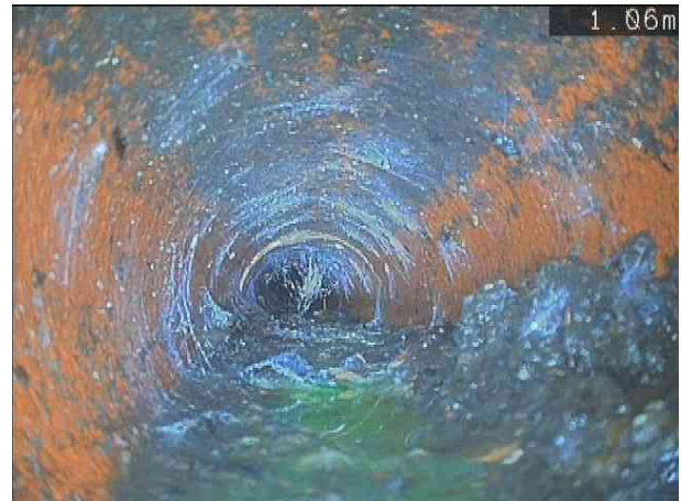
RWWG1X_24ee1754-99c7-49c4-b9b0-5a0b47d49434_20241106_122018_704.jpg, 00:00:36, 1.06 m Settled deposits, fine, 25% cross-sectional area loss, start
