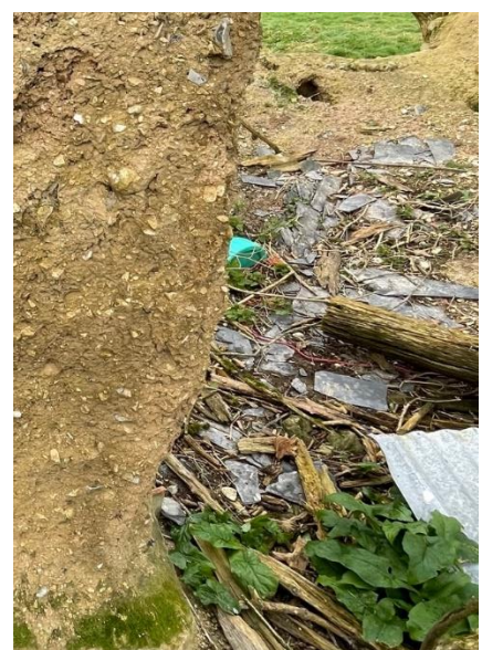
Evidence of slate roofing on barn floor
