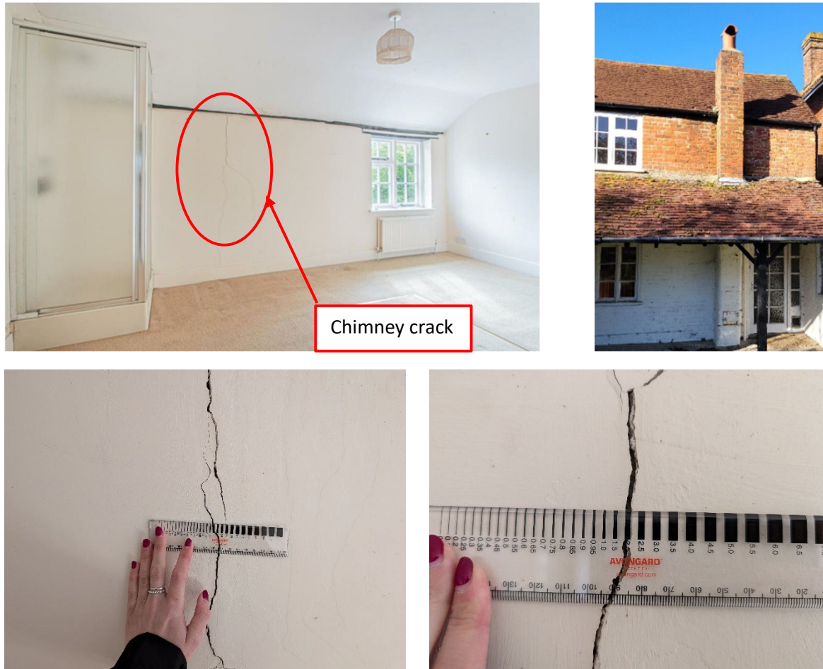
Figure 6 showing position of crack (internally/externally)
