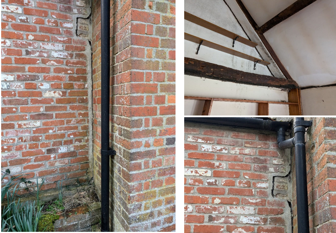
Figure 9 showing corner separation between rear extension and house
