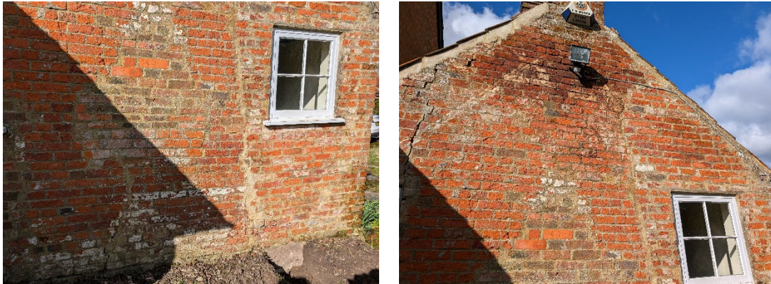
Figure 7 showing cracking externally to rear elevation.
