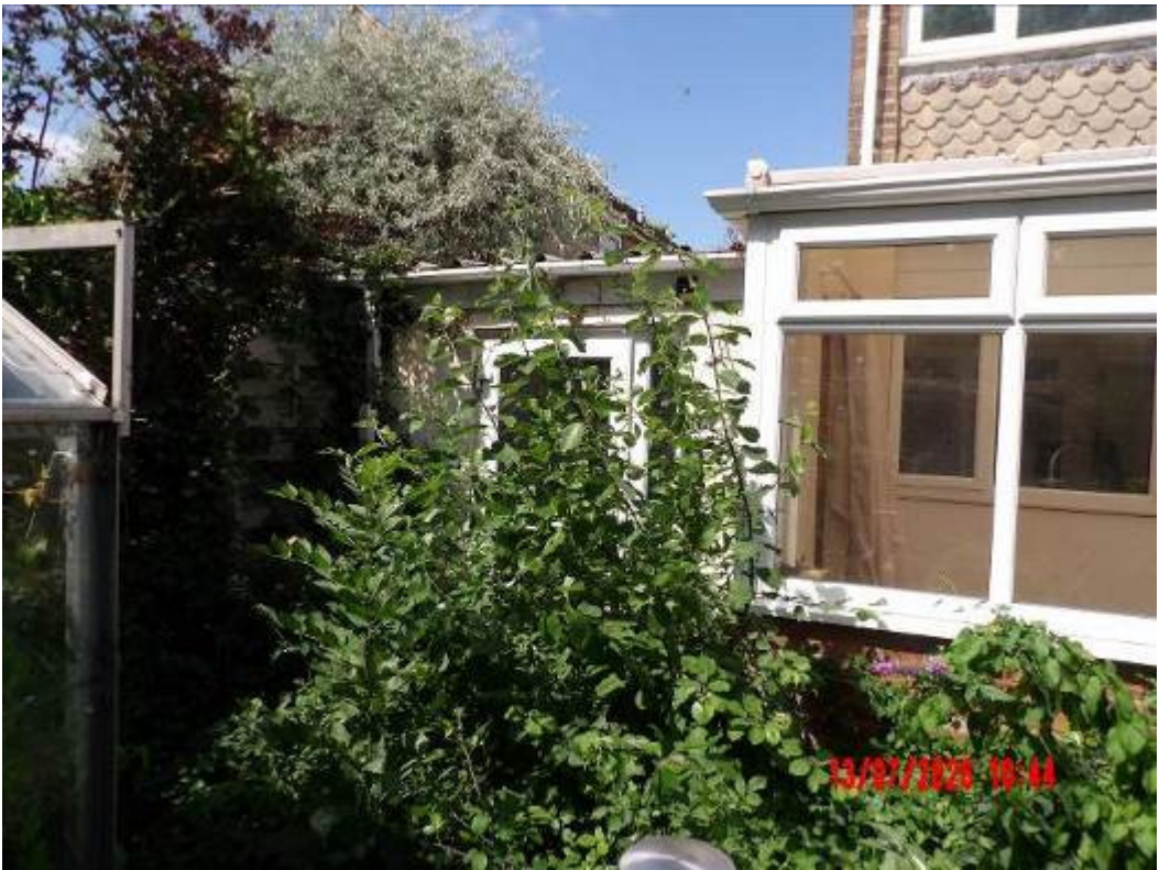
6. PARTIAL REAR ELEVATION SHOWING EXCESS SHRUB GROWTH.
