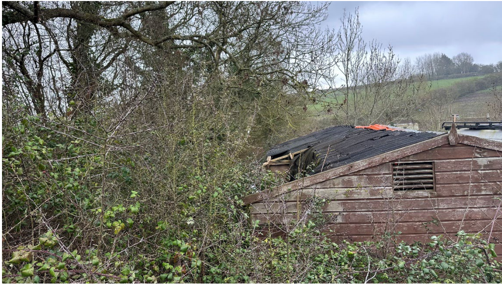
Plate 11: The roof has collapsed in areas.
