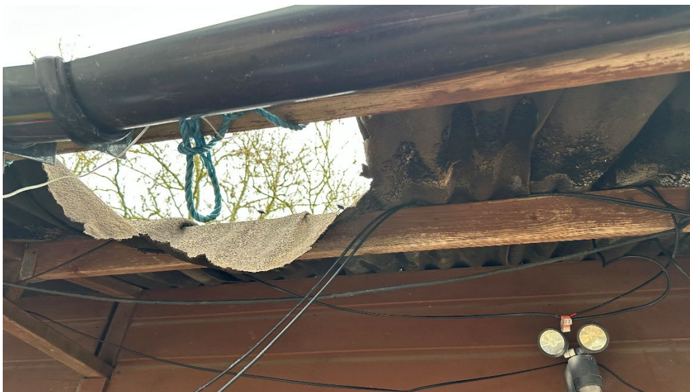
Plate 10: The stable building is in a state of disrepair.
