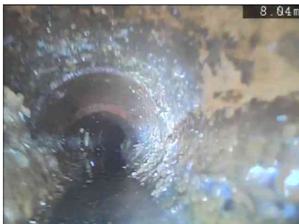
WG1X_d2b3d92d-5d2f-4ae0-95b3-ab1038b4e698_20241121_115526_427.jpg, 00:01:29, 8.04 m Debris, other, 15% cross-sectional area loss, Sludge
