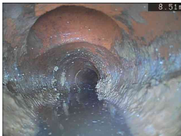
WG1X_05d1a62b-3793-41c4-bf1b-ae873b1d2594_20241121_115544_085.jpg, 00:01:32, 8.60 m Junction at 12 o'clock, 100mm diameter
