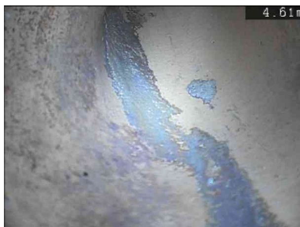
SVP1X_f82cc0eb-303f-4990-85ef-8a8e4e07672b_20241121_1 14918_286.jpg, 00:00:23, 4.61 m Line of sewer deviates up, Rest bend
