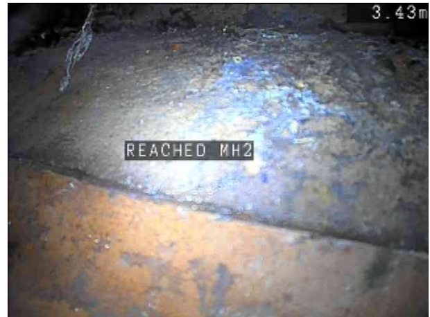
MH1X_84a04fb6-ebdf-4e08-bb8d-6de8cb671c68_20241121_1 15036_757.jpg, 00:00:40, 3.43 m Finish survey, Reached MH2
