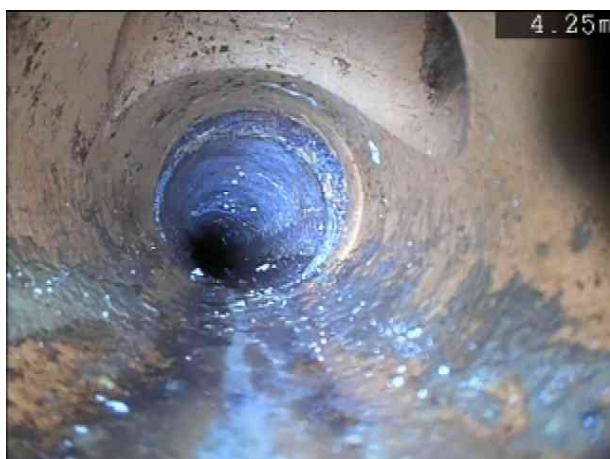
WG1X_5ae9ce26-e4d2-4bbf-83bc-82025ba7ce8e_20241121_115319_013.jpg, 00:00:56, 4.30 m Junction at 12 o'clock, 100mm diameter
