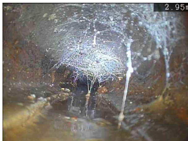
MH2X_83ed2d8c-00c5-405c-a74f-aaf52ac2fdb8_20241121_120135_798.jpg, 00:00:33, 2.95 m Debris, grease from 4 o'clock to 8 o'clock, 15% cross-sectional area loss
