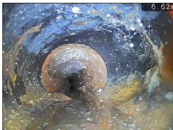
WG1X_4bff2193-5657-471e-8e58-5ac0504a20e9_20241121_115425_829.jpg, 00:01:17, 6.62 m Junction at 3 o'clock, 100mm diameter
