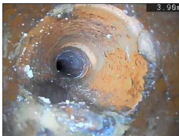
WG1X_28c188eb-0d7b-46e3-8c54-585fb1c6387e_20241121_115643_279.jpg, 00:00:47, 3.90 m Scale, medium at joint from 4 o'clock to 8 o'clock, 15% cross-sectional area loss
