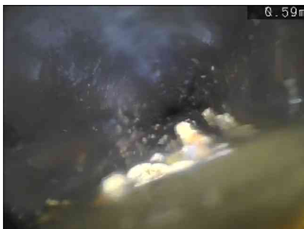
SepticTankX_5f9b4a6d-f3c4-4fd8-994f-b6769e08f054_20241121_114236_609.jpg, 00:00:46, 0.59 m Debris, other, 20% cross-sectional area loss, start, Loose
