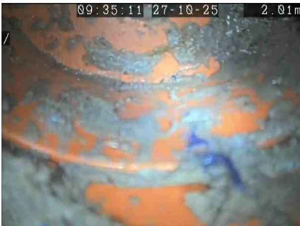
a9f9bf08-3cd1-42fa-b145-120fe4f23540_1_1.png, 00:00:38, 2.01 m Finish node, manhole, reference: WC
