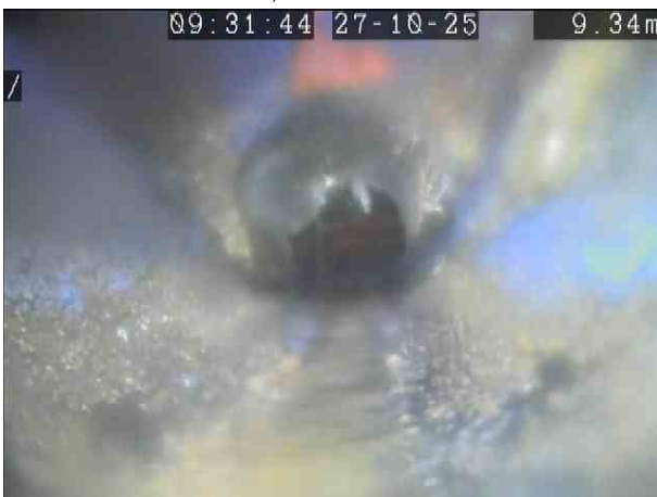
4dd0f1a3-013c-46fc-863e-f8f79428b4f8.png, 00:00:43, 9.34 m General remark, MH4 THROUGH MANHOLE
