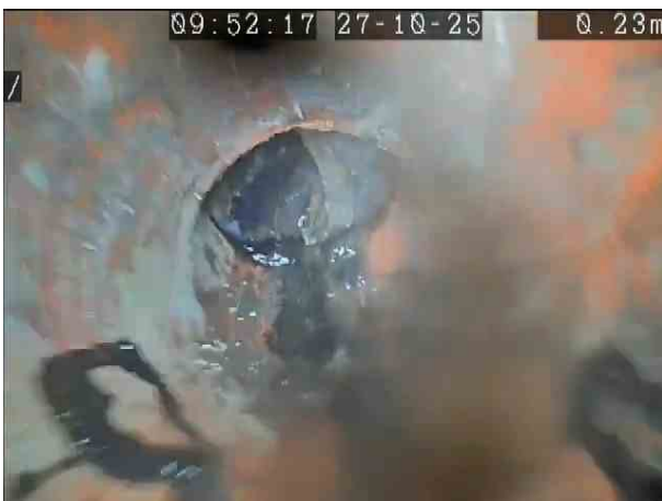
d9e60f67-580e-42dd-902c-660e65af7d8f.png, 00:00:34, 0.23 m Joint displaced, large
