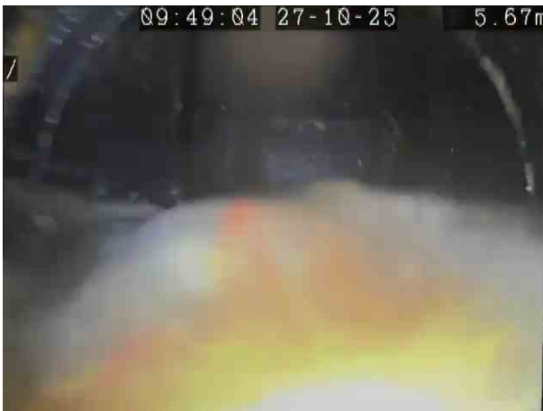
f1cc4df8-06e3-438d-9c03-e0be9aaa52fd.png, 00:01:59, 5.67 m Attached deposits, grease from 4 o'clock to 8 o'clock, 20%
