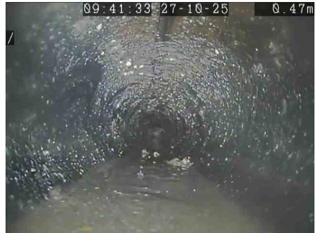
f6fc9649-c0df-4c5c-85c3-4e7f7474a6b6.png, 00:00:13, 0.47 m Attached deposits, grease from 4 o'clock to 8 o'clock, 20%
