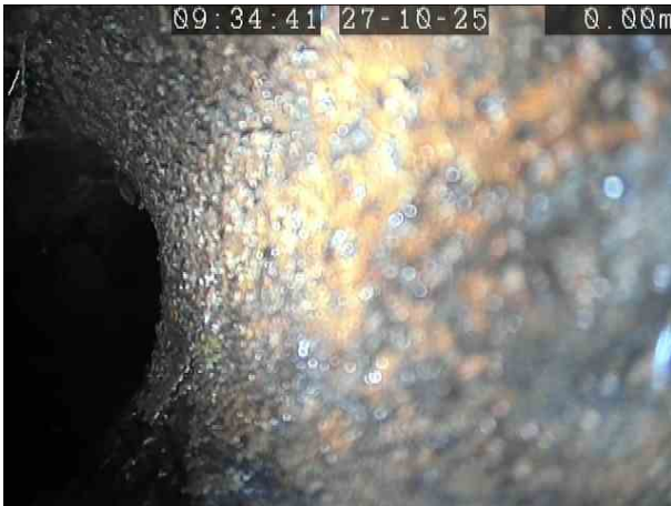
7282af5e-59f1-4a53-8e55-6f033a7ed371.png, 00:00:08, 0.00 m Start node, manhole, reference: VC2
