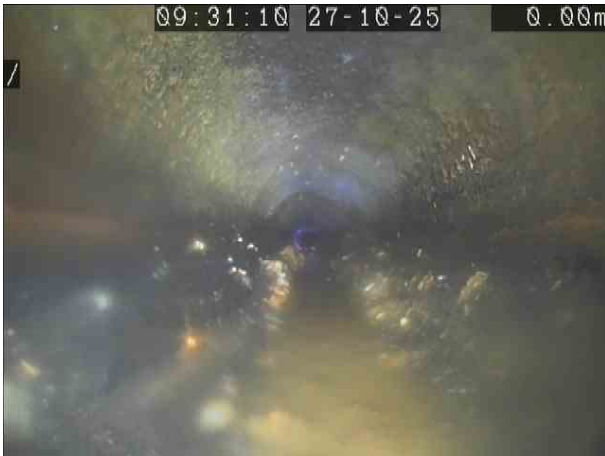
85920f19-b7e9-4bf4-8d79-197a73841a81.png, 00:00:09, 0.00 m Start node, manhole, reference: I/C1
