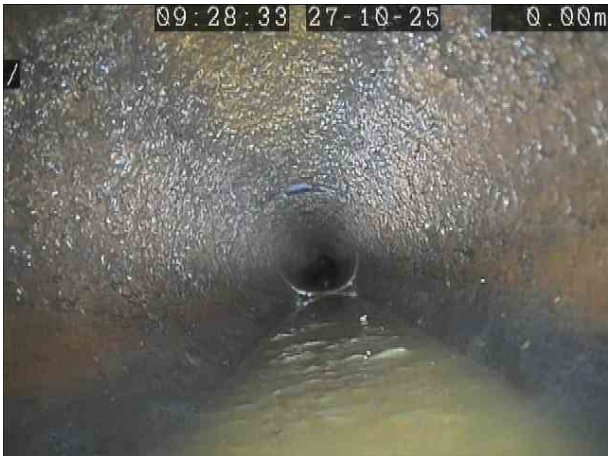
caeec61f-4d90-4d13-af23-26eabea73880.png, 00:00:18, 0.00 m Start node, manhole, reference: /C1
