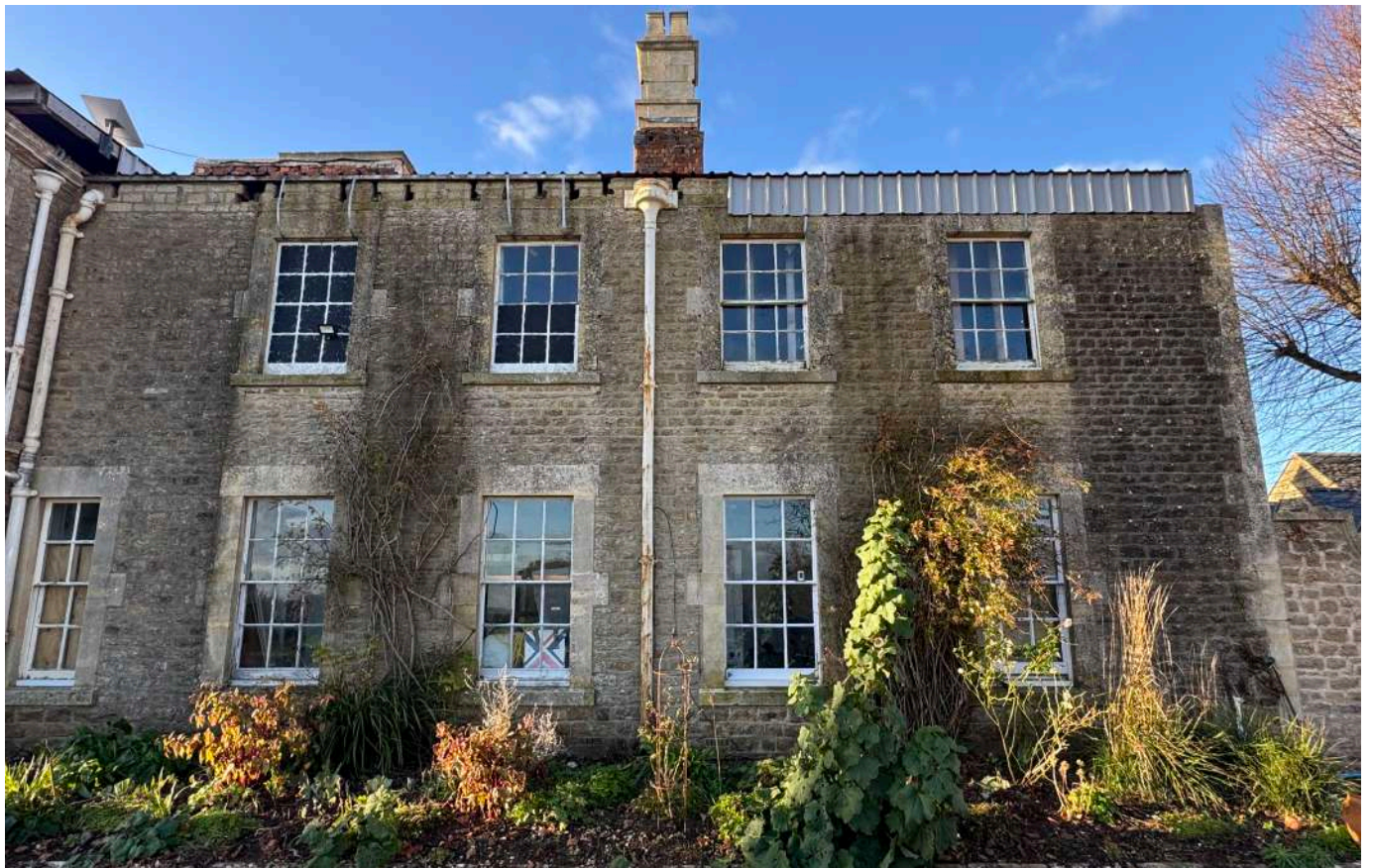
Figure 5.4: East Wing South Elevation, post-fire
