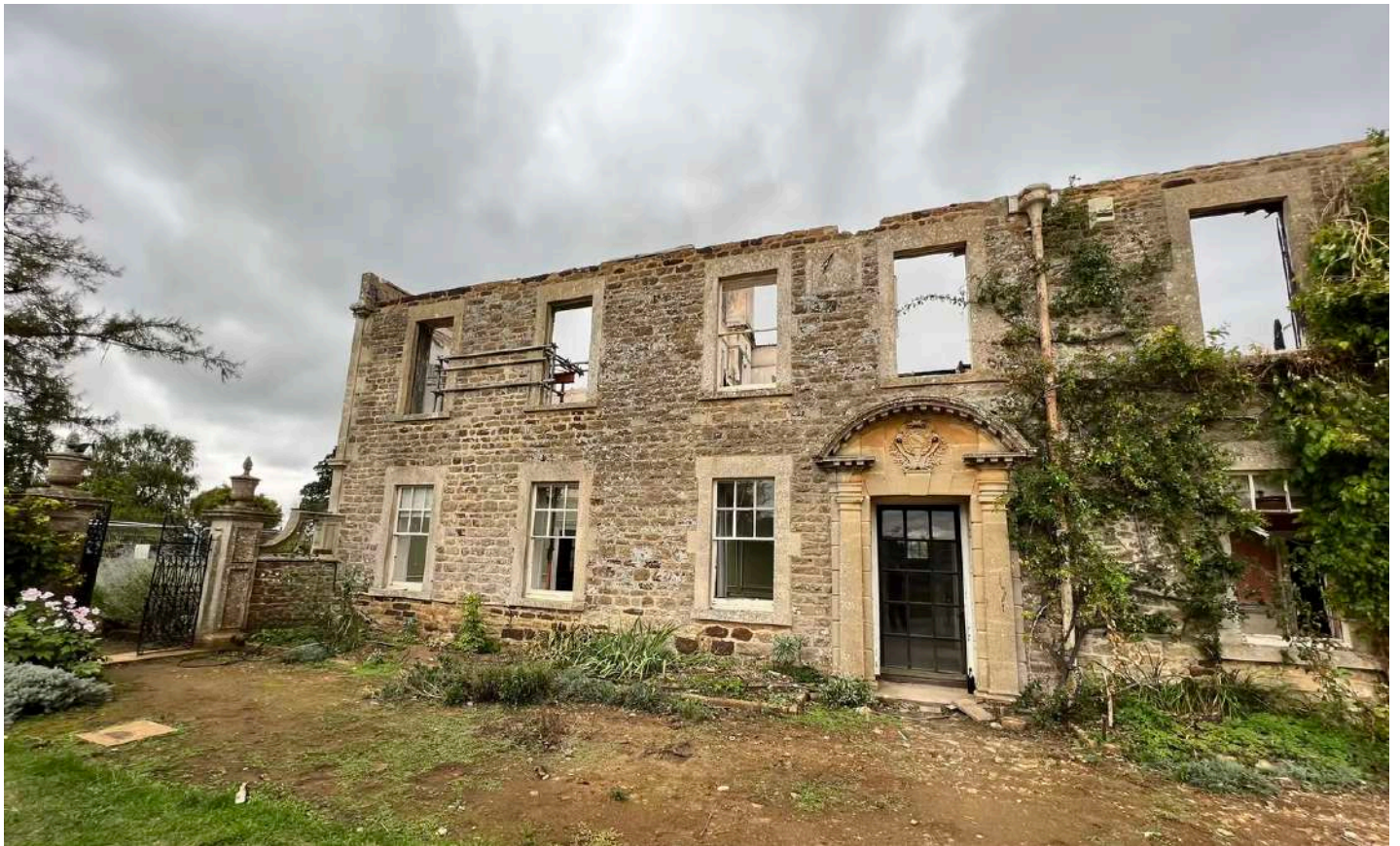
Figure 5.3: Nonsuch House, South Elevation. Fire-damaged shell
