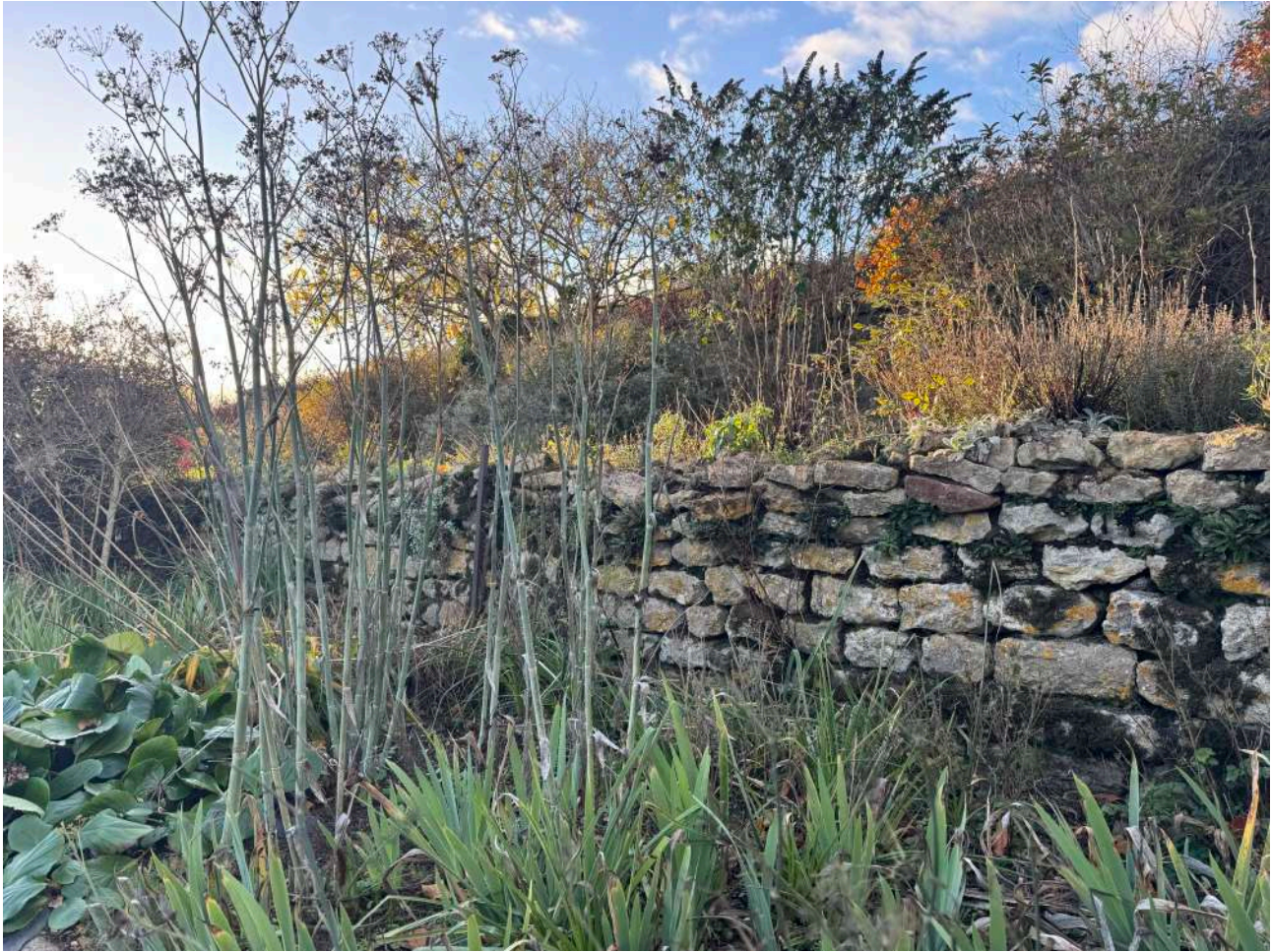
Figure 5.9: Raised terrace in Larch Garden - condition of wall
