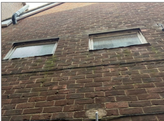
Figure 17 - Window on south elevation to be enlarged
