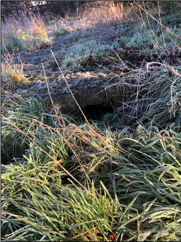
Photograph 10: Mammal hole underneath concrete platform.
