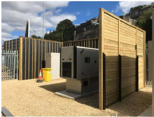
Example of absorptive acoustic timber fencing around plant area. Jackson Jakoustic Absorptive 2.0m high or similar approved, with the potential for upto a 32dB reduction in noise.
