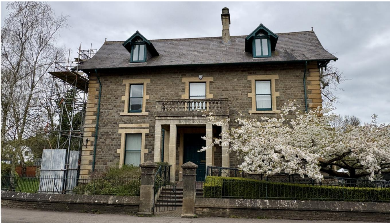
Fig.2: Bank House front elevation, with scaffolding to the affected southwest elevation on the left (via historic England)
