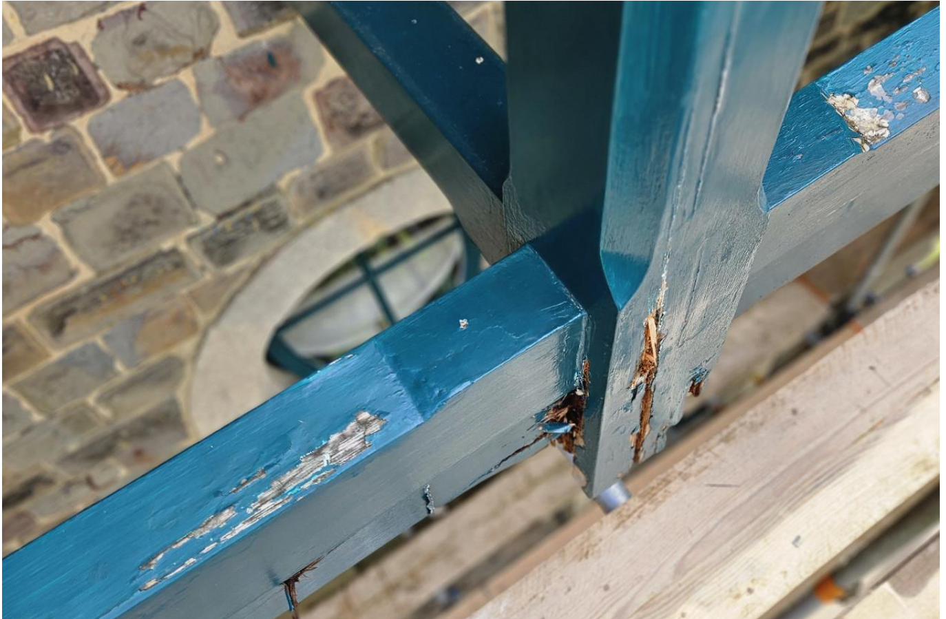
Fig.4: Damage to timber pendants and tie-beam to gable end
