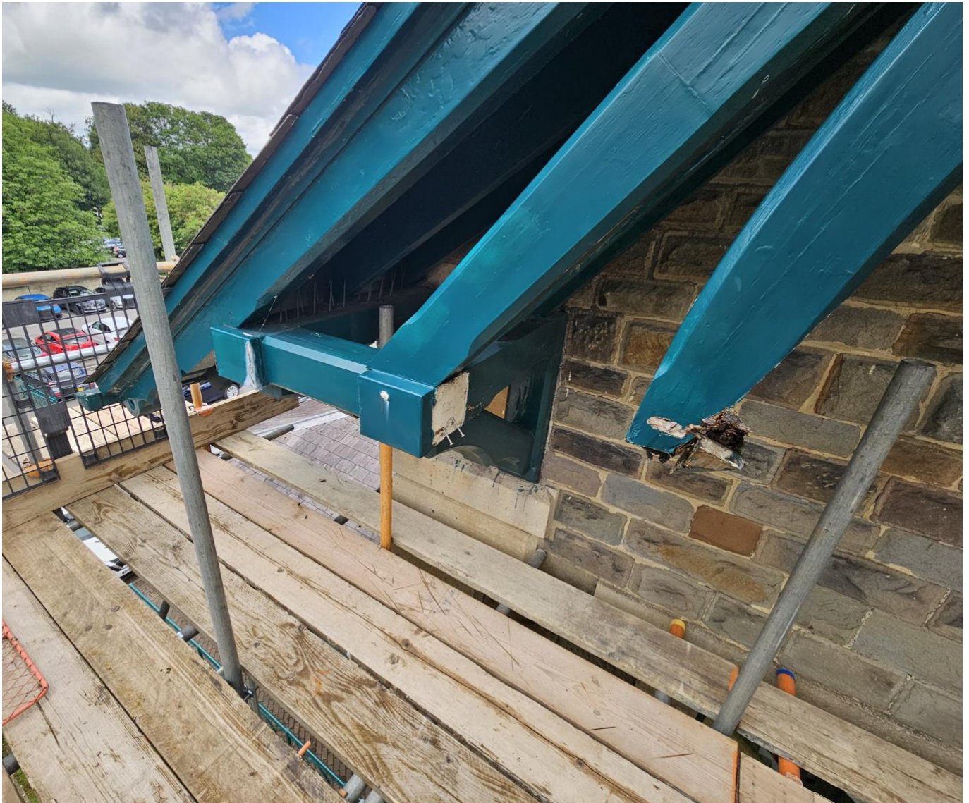
Fig.3: Damage to bottom of archbrace and missing finial section
