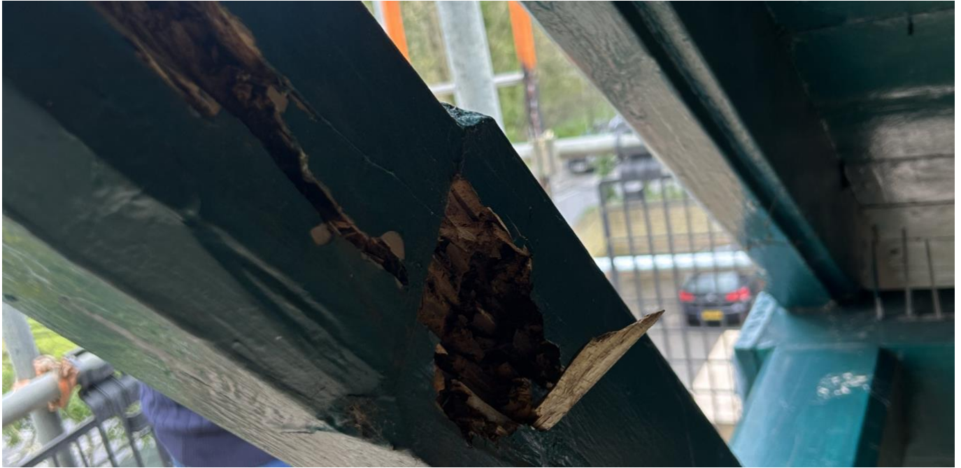
Fig.6: Damage to archbrace
