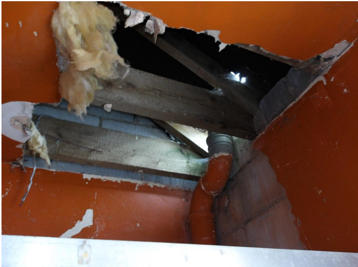
Photograph 3: showing roof & loft space with a gap (potential bat access/egress point)
