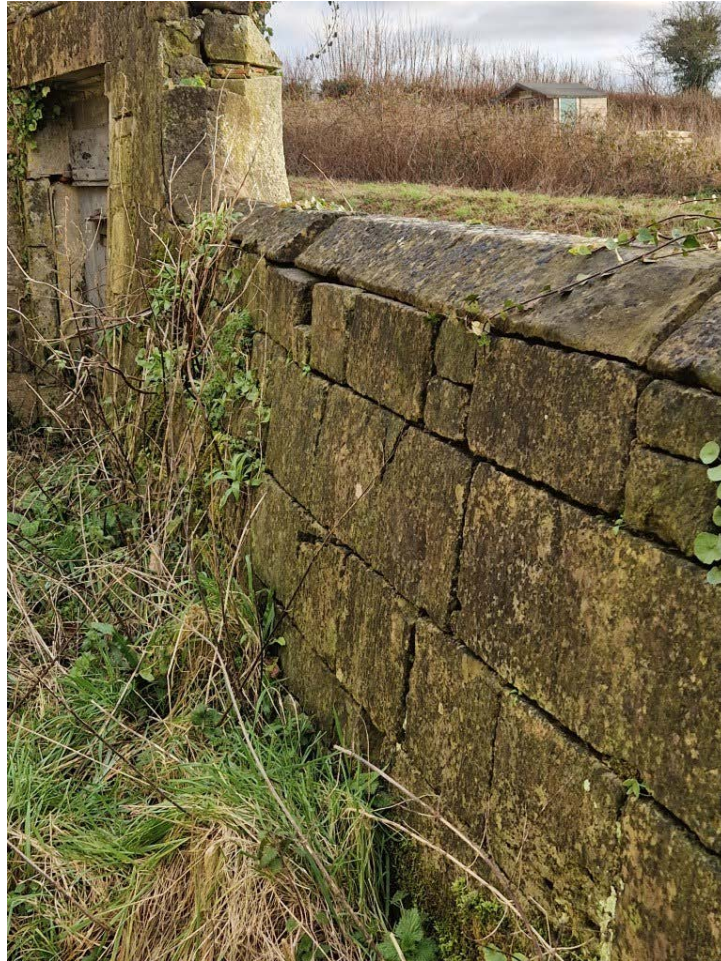
Photo 3: Displacement and leaning of the coursed stonework, consistent with ground movement beneath the wall's foundation.
