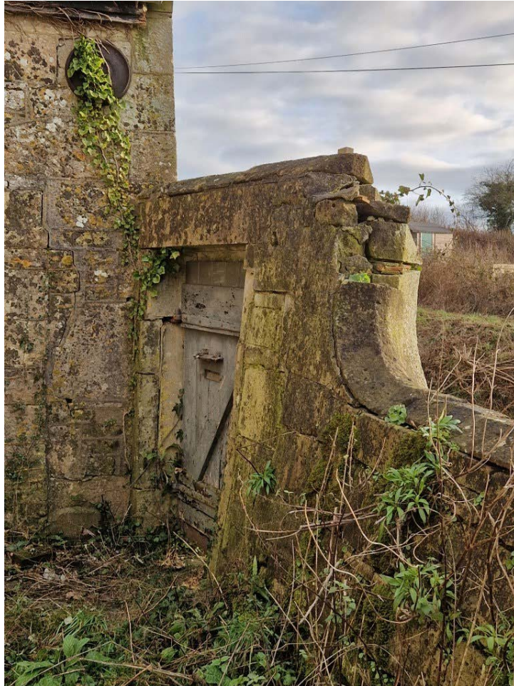
Photo 4: Cracking and displacement of the stone coping at the gated entrance pier, showing the extent of movement.
