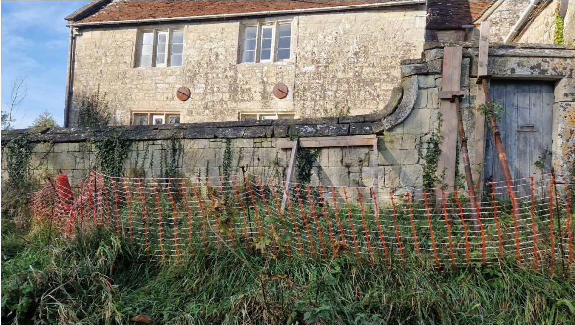
Photo 1: General view of the boundary wall and subsidiary rear gated access from the roadside, showing its relationship to the farmhouse and the temporary propping currently in place.
