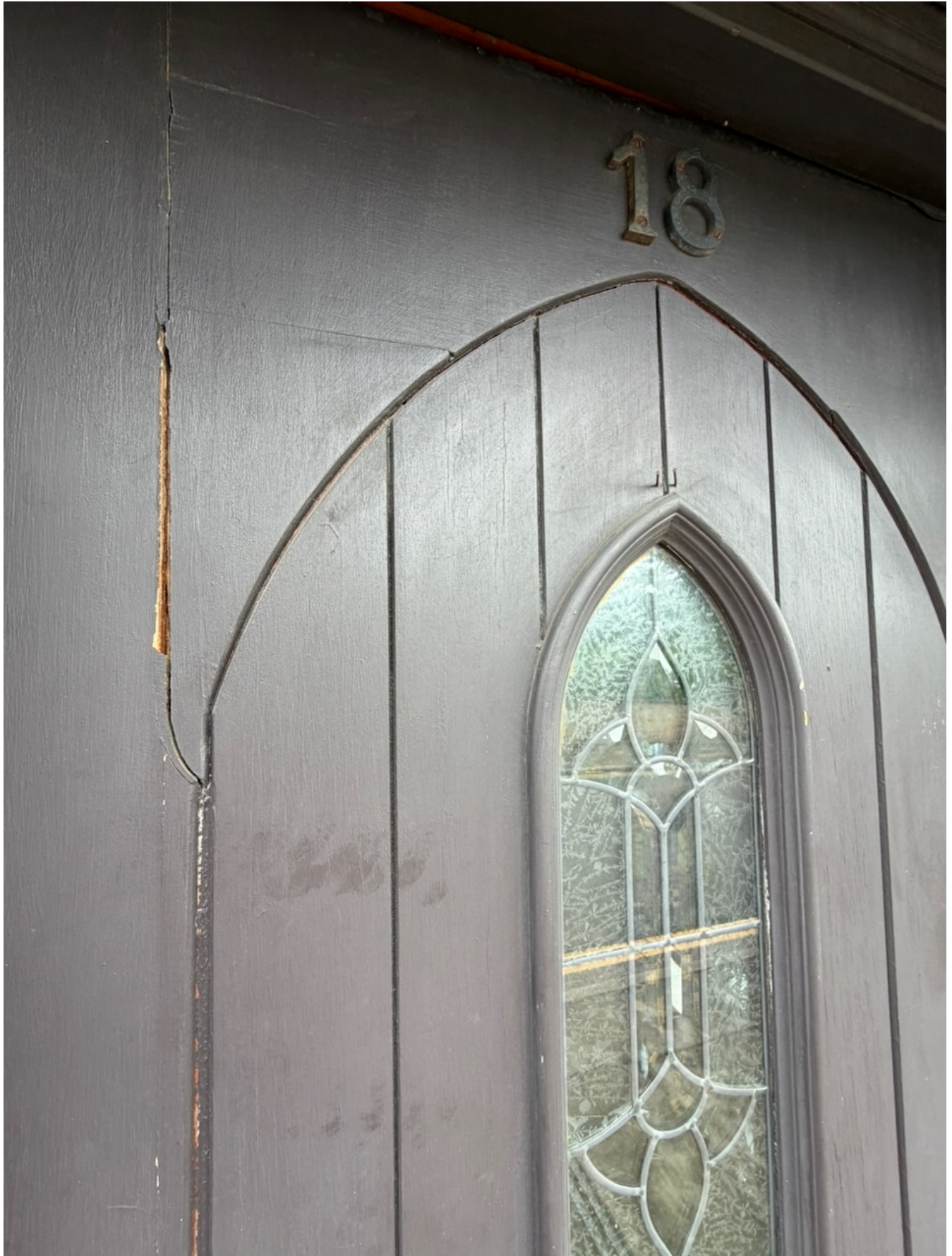
Photograph 3: Deterioration of current door
