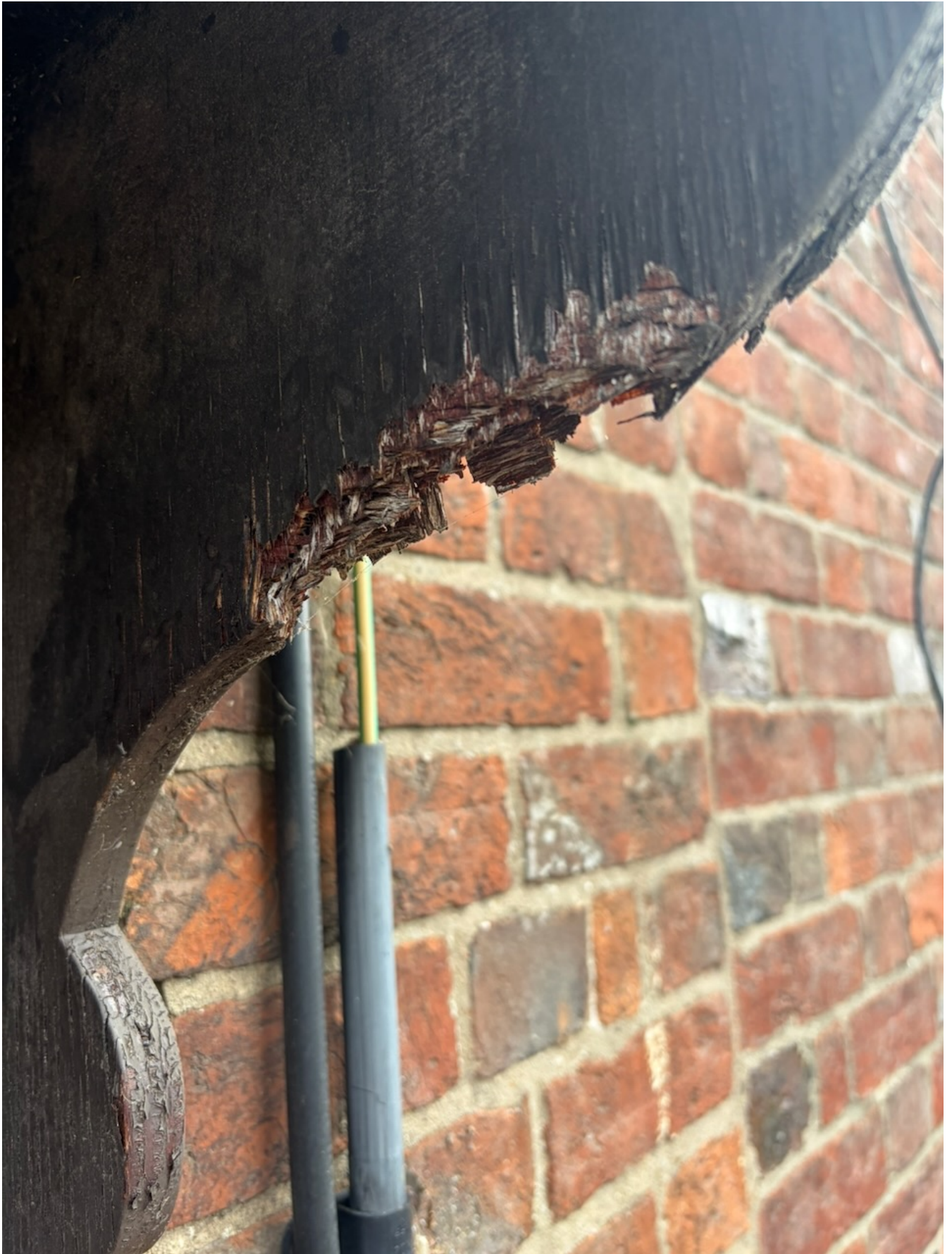
Photograph 5: Deterioration of canopy
