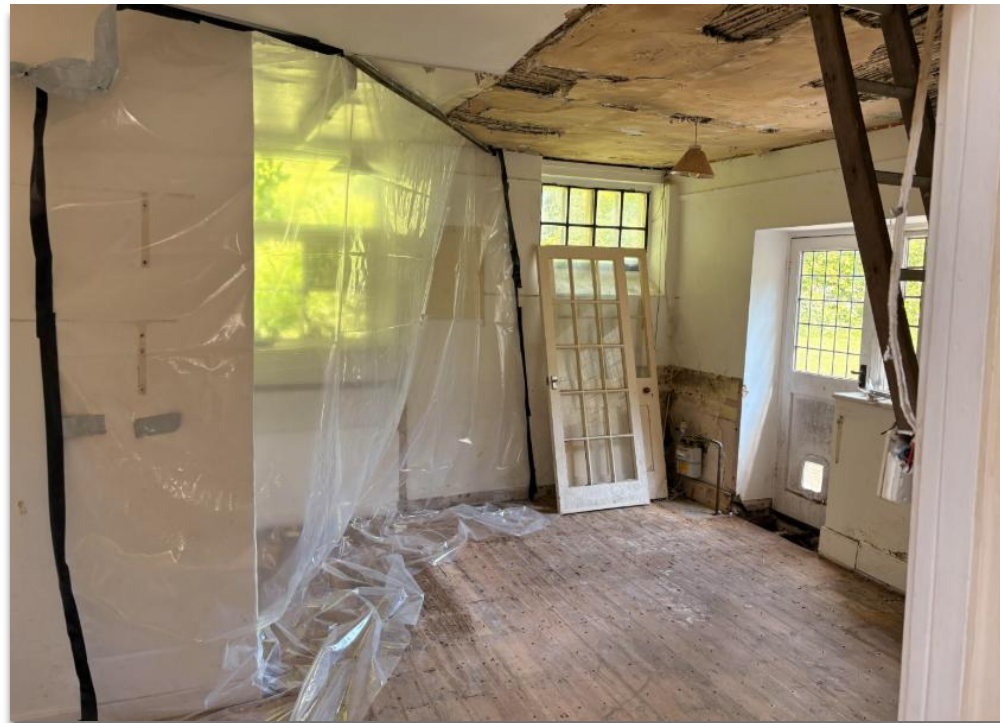
Figure 1. Proposed kitchen. Note fibreboard partition with modern skirting boards, and cracked, blown and dropping plaster from lathes, and C20 pine floor.
