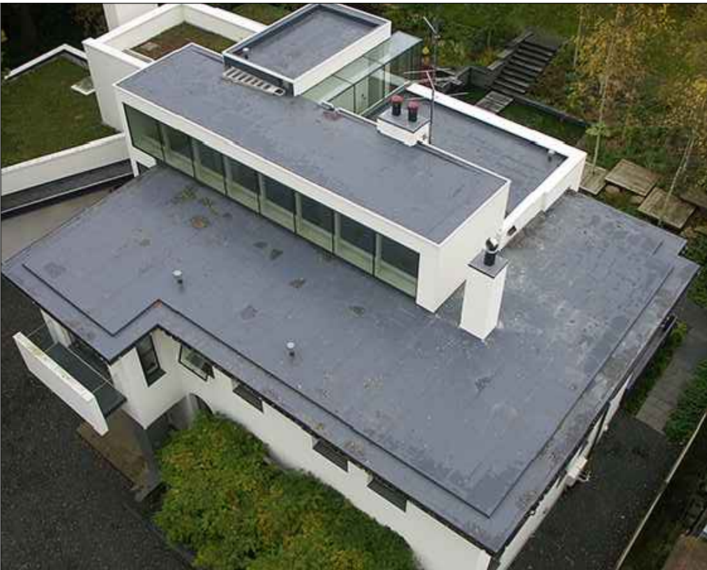
Flat Roof - ICB Group Alwitra Evalon VSK single ply membrane Slate Grey
