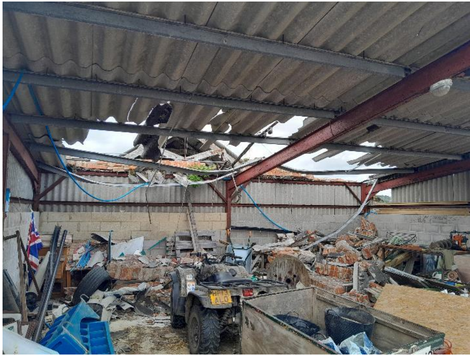
Photo 20. Inside B9, showing partial roof collapse.
