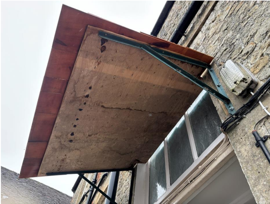
Fig.5 Canopy over the back door cutting across the fanlight
