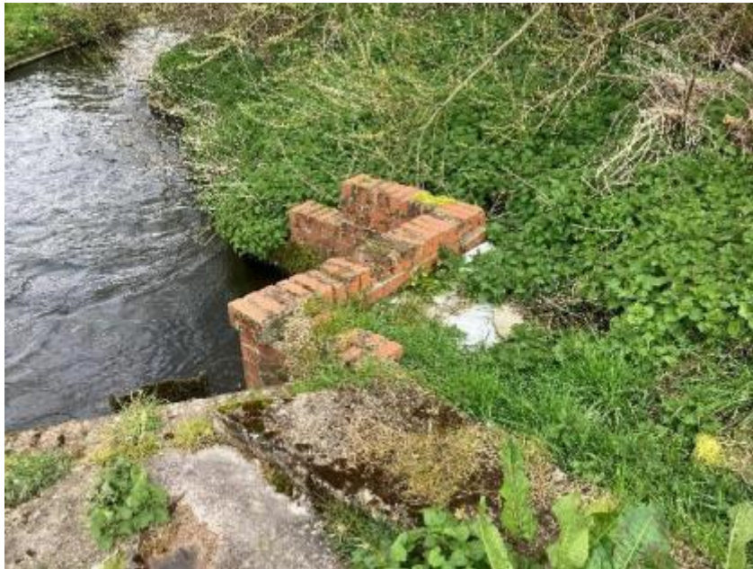
Figure 4: Section of Headwall to be repaired and missing bricks replaced like-for-like.
