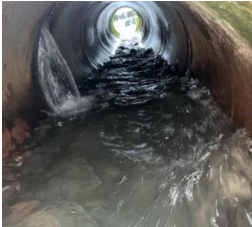
Figure 5: Leak within the culvert through culvert barrel jointing
