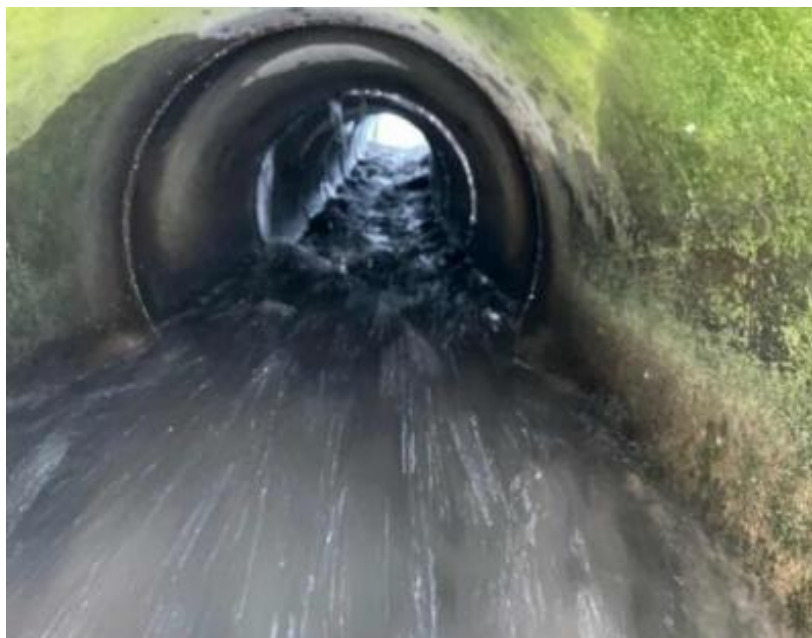
Figure 6: Multiple leaks through culver barrel jointing
