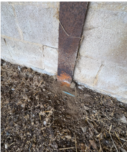
Example of surface corrosion at column base in B2
