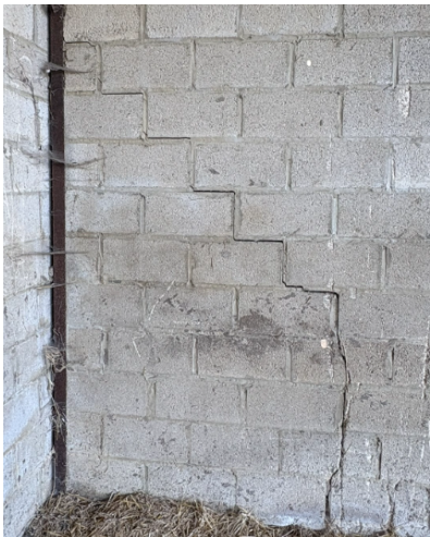
Diagonal crack in B2 requiring helibar repairs
