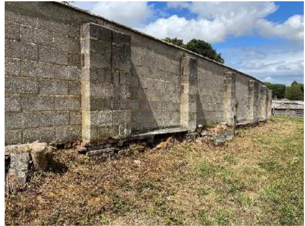
Figure 3 – Undermining of retaining element to Wall B
