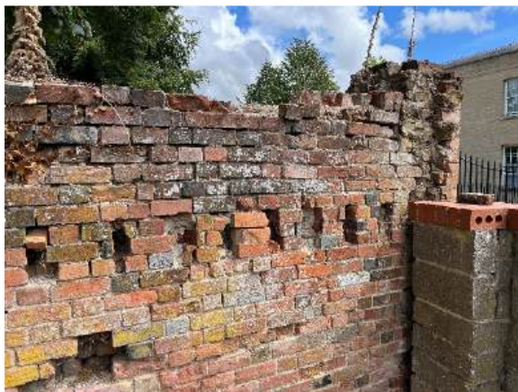
Figure 4 – Deterioration to Wall G
