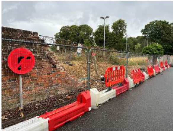
Figure 2 – Collapsed Section of Wall E
