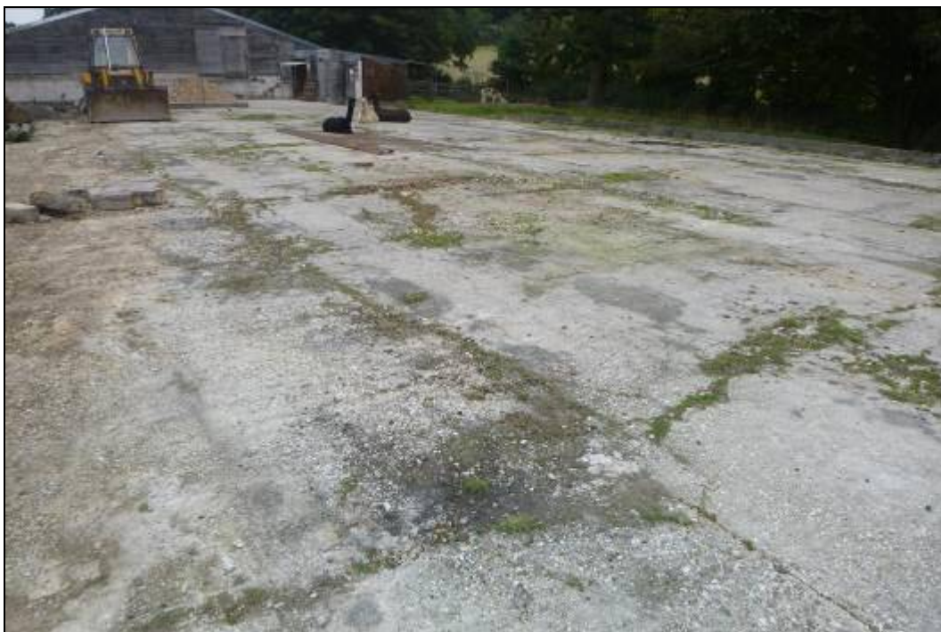
Photograph 8 Showing the condition of the concrete base
