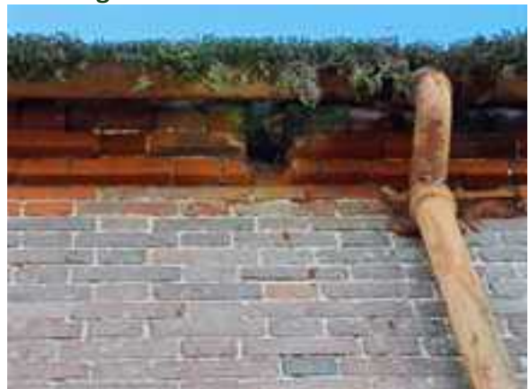
Figure 56: A missing eave brick to the left of the gutter on the east elevation of the main dwelling
