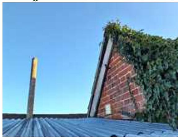
Figure 50: Gap under the rake/fascia board on the northern elevation of residential dwelling's extension
