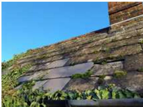
Figure 49: Loose slate tile on the west elevation of the residential dwelling's extension
