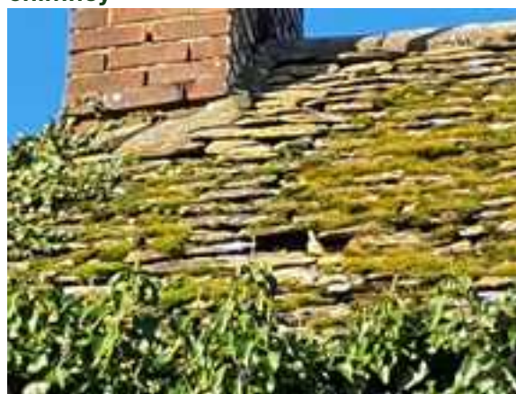
Figure 62: A raised tile on the south facing pitch of the main roof and near the eastern chimney
