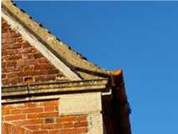
Figure 57: Cracked mortar on the south-east corner of the main dwelling's roof
