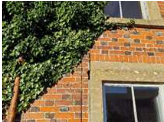
Figure 60: Gap in the wall mortar around the ground floor window lintel beam
