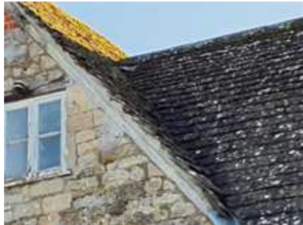
Figure 54: An example of a roof valley with multiple inherent gaps under the stone tiles
