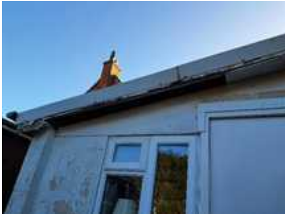
Figure 51: A missing soffit board on the northern elevation of residential dwelling's extension
