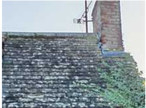
Figure 52: Raised flashing around the western chimney and inherent gaps in the stone tiles
