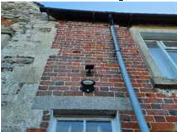
Figure 55: A missing eave brick under the to the right of the gutter on the north elevation of the main dwelling
