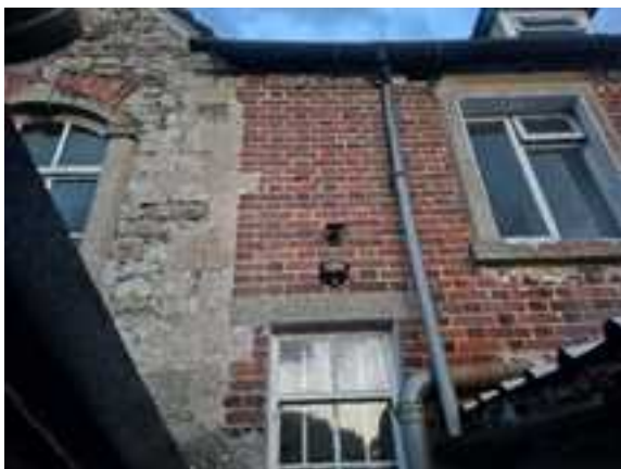
Figure 73: A light fitting on the north side of the main dwelling positioned high on the wall
