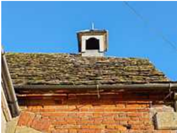
Figure 59: Another view facing east of the belfry along with the inherent gaps in the natural stone tiles
