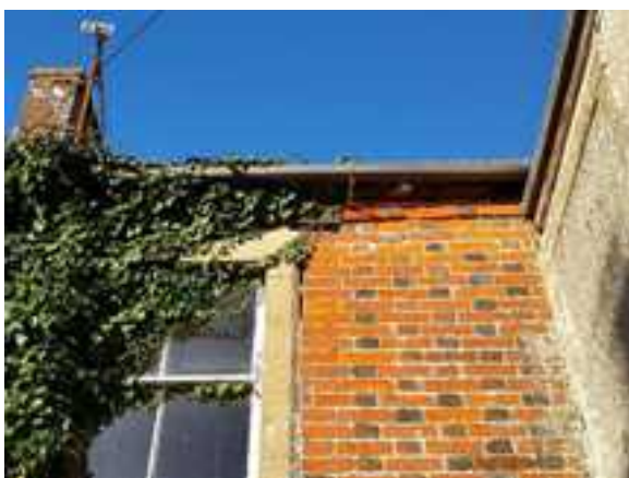
Figure 61: Gap in the wall mortar around the window of the first floor
