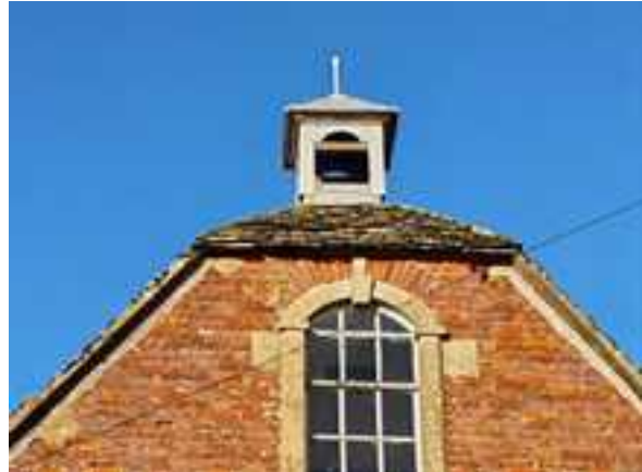
Figure 58: Inherent gaps in the natural stone tiles
