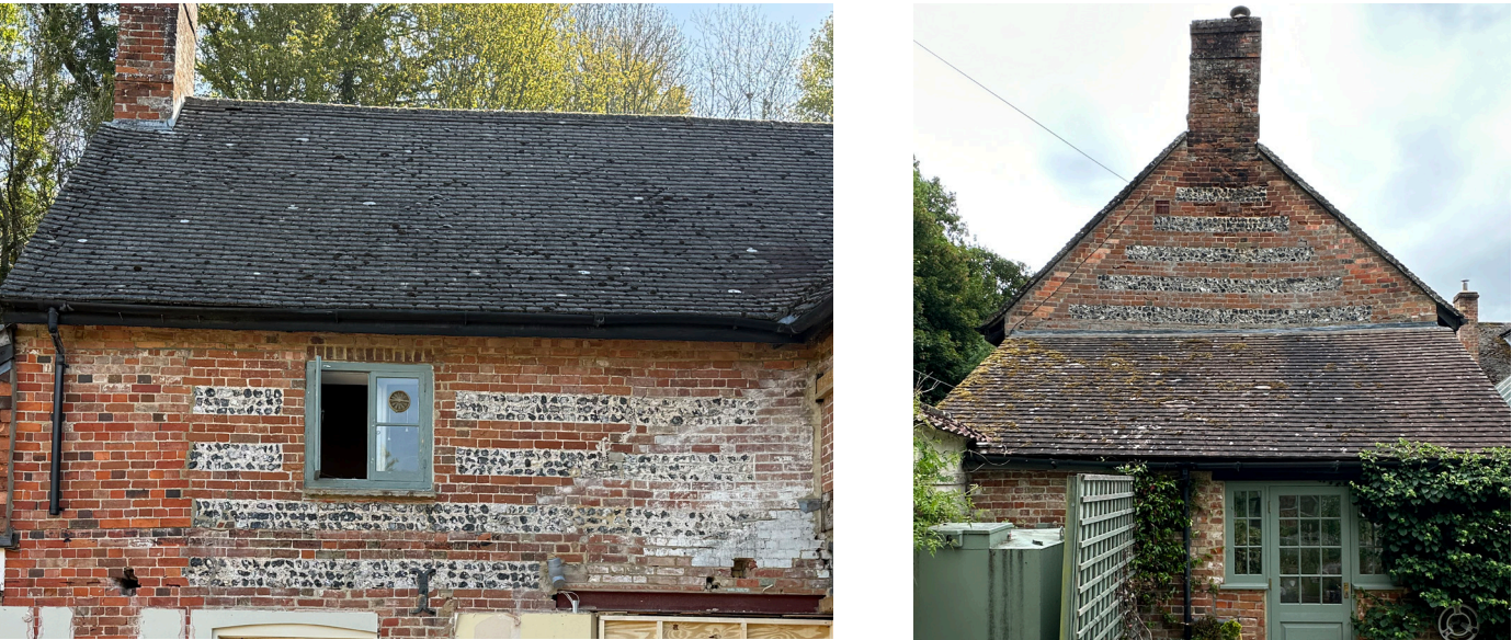
Images: Evidence of extra brick coursing below the eaves and on the gable end verges to mask the subsidence.
