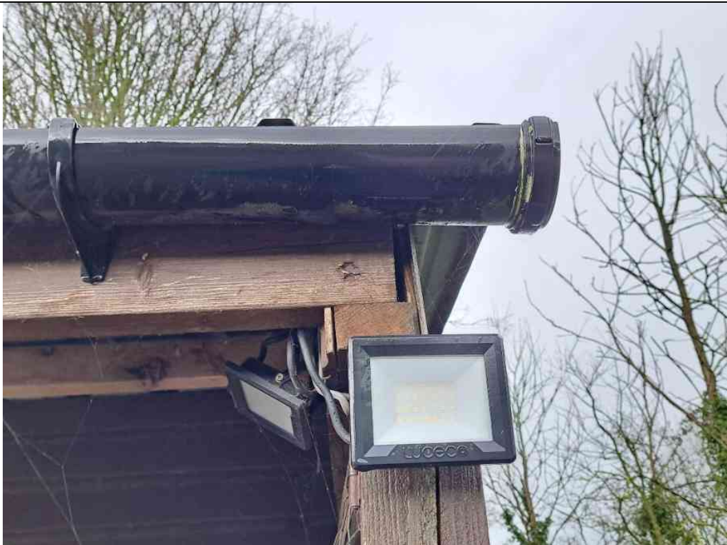
Gap at side of fascia board on west elevation of Active Stable
