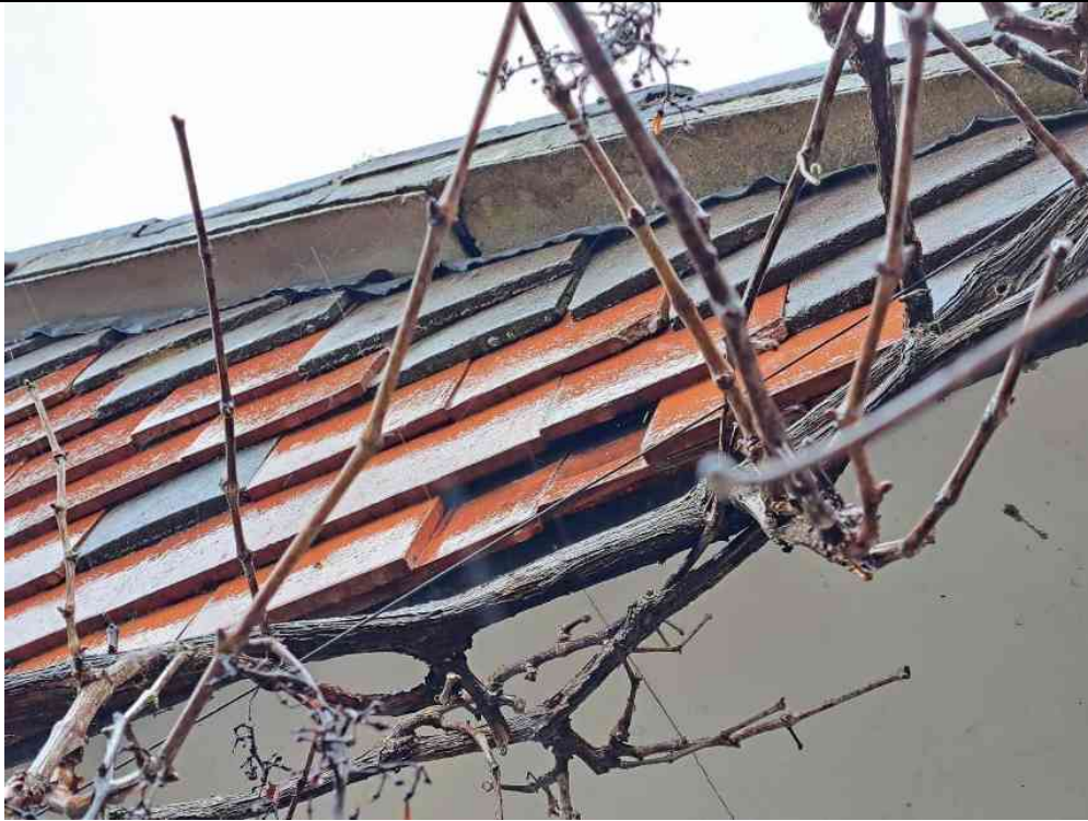
Gap where vertical wall tile is missing on southern elevation of Disused Stable
