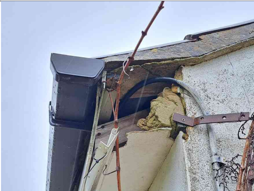
Hole where end of fascia board is missing at south-west corner of Disused Stable
