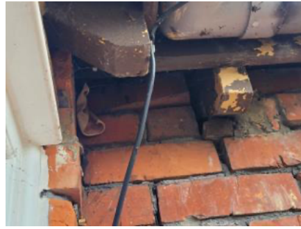
Photo 4: Loose brickwork around exposed rafter tail.
