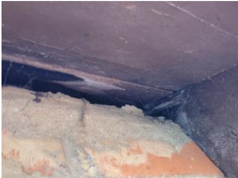
Photo 5: Gap between the wall top and roof.
