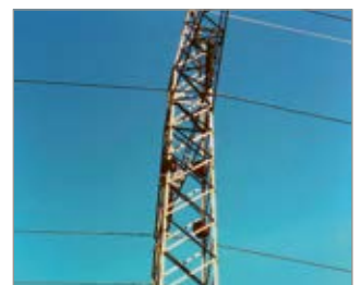
▲ Installation example on a power pole
