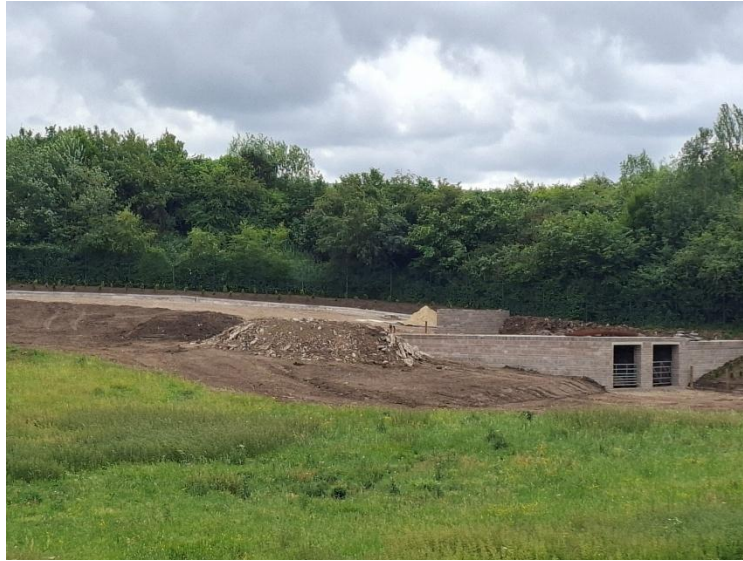
Fig 1: Construction as at 2 nd June 2026. All features are unauthorised.
