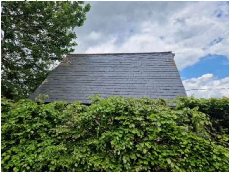
Photograph 5: Gaps between slates
