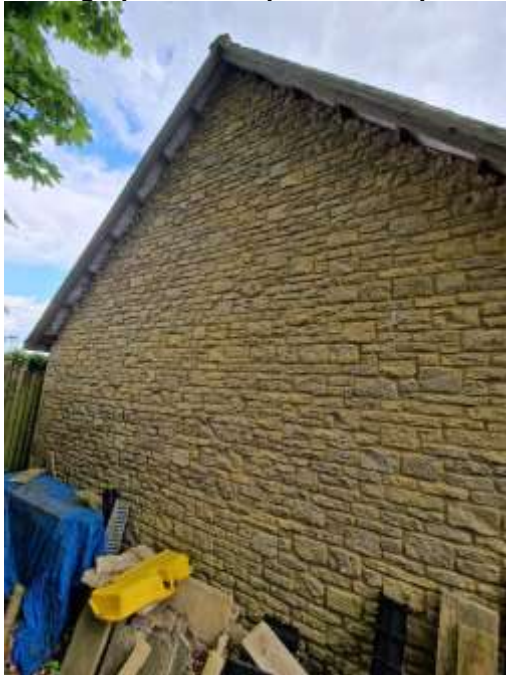
Photographs 6-7: Gaps in wall tops
