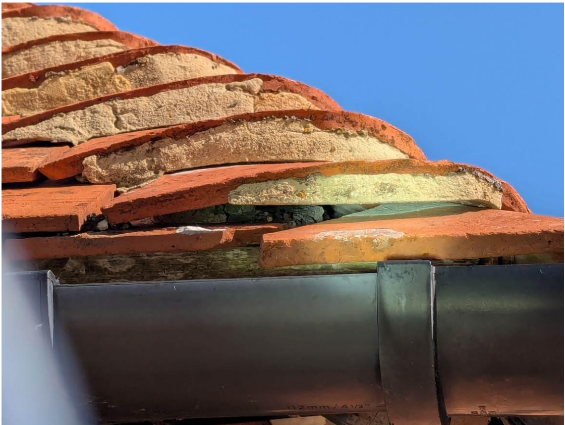
Photo 7/8 The Old Livery, (south aspect) tile clay roof tiles gap and high potential feature tile gaps
