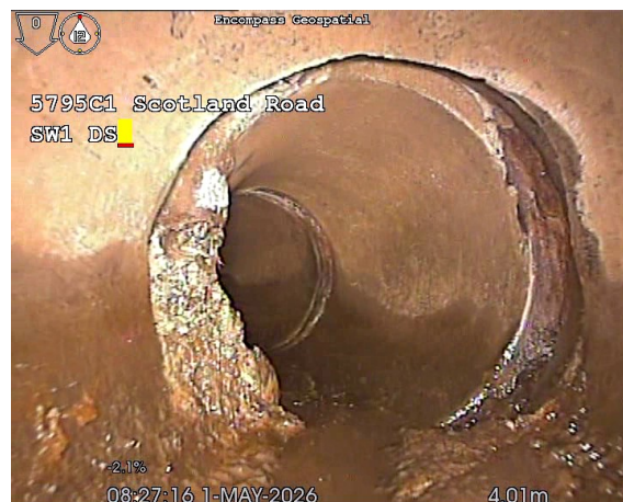
SW1X_22024b9f-98b7-4a9e-9673-4d2d928e13b0_20260511_100016_121.jpg, 00:00:26, 4.01 m Open joint, medium
