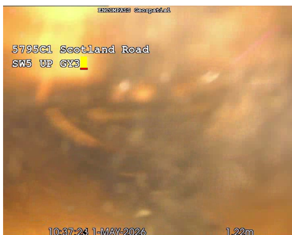
GY3X_767c2f35-07b0-4543-aaba-97f7f7b4e1bd_20260511_10 2228_702.jpg, 00:00:04, 1.22 m Joint displaced, medium
