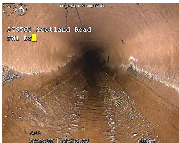
SW1X_cca77ac0-2b28-43e5-941e-e3228ee24f81_20260511_095940_180.jpg, 00:00:00, 0.00 m Settled deposits, fine, 5% cross-sectional area loss, start
