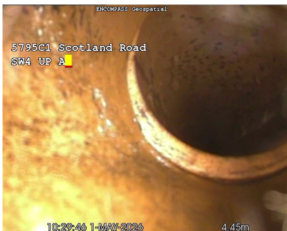
SW5X_5de816cb-a3b1-47db-9a60-9a4c93cc8d9a_20260511_101913_661.jpg, 00:00:42, 4.45 m Joint displaced, medium
