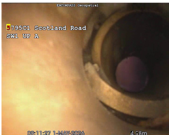
SW1 UP AX_1319379e-1f4b-403f-afbe-5195f6e8edd5_20260511_10041 2_262.jpg, 00:00:20, 4.98 m Joint displaced, large
