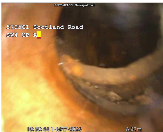
SW5X_464c6baf-bd51-4aec-9b69-e566cd002e00_20260511_102038_147.jpg, 00:01:40, 6.47 m Survey abandoned, UNABLE TO SURVEY OVER THE JOINT
