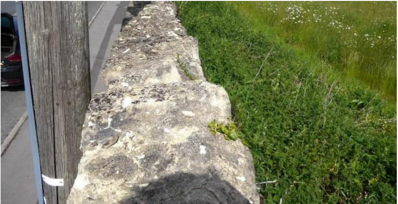
Severely eroded wall copings
