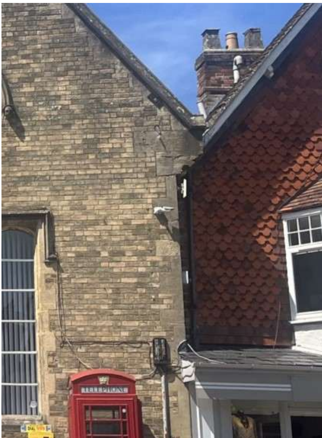
Location of existing CCTV camera
