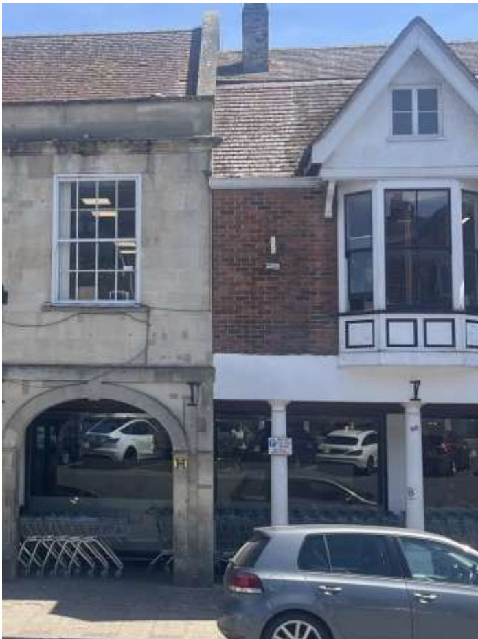
Location of existing CCTV camera on brickwork
