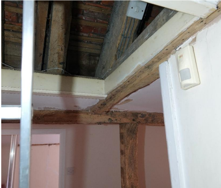
Fig.133 The foot of T2A showing how it is misaligned in relation to the adjacent post, but does have a thin tiebeam running back to the stack
