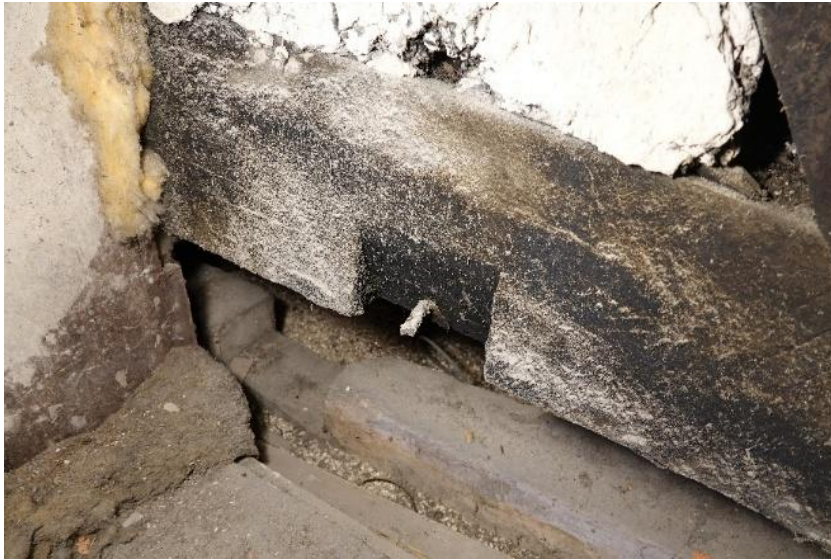
Fig.122 The collar of T2, showing the vacant open mortise with its iron nail
