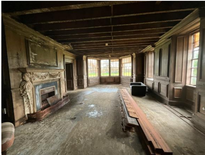
Figure 3: Existing state of disrepair in the 'Music Room' following the fire
