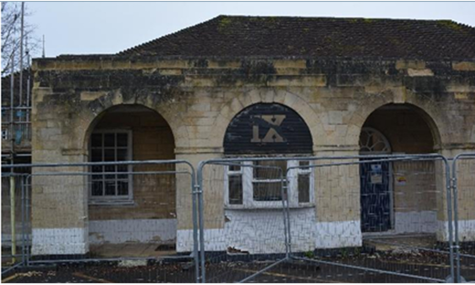
Façade (North East Elevation), Showing Extent of Stonework Spalling, 2026
