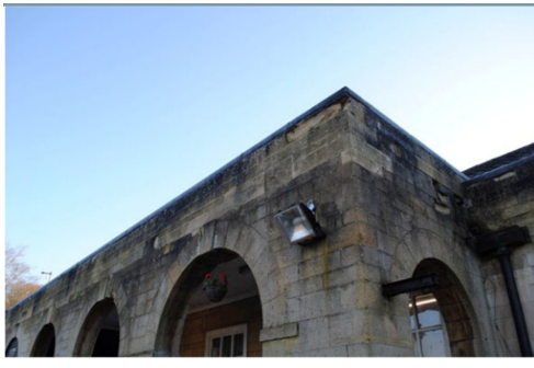
Northeast Parapet, Showing Spalling Stonework, 2020
