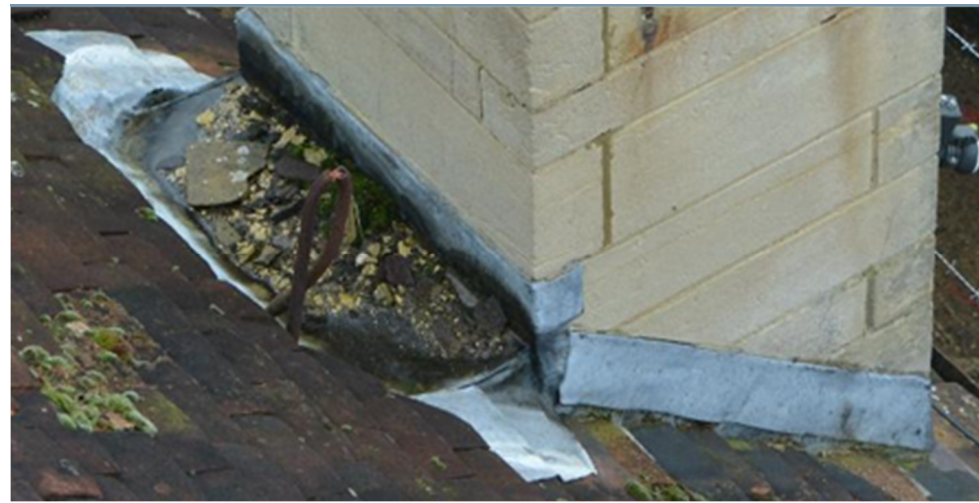
Chimney Stack Back Gutter and Side Flashing, 2026
