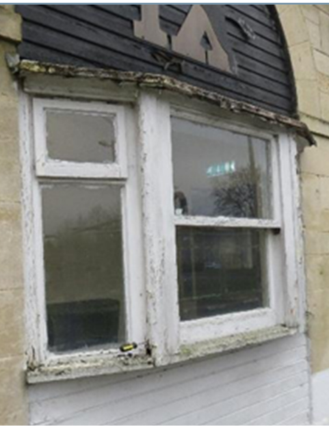
Façade Oriel Window, Showing Rotten Timbers, 2026
