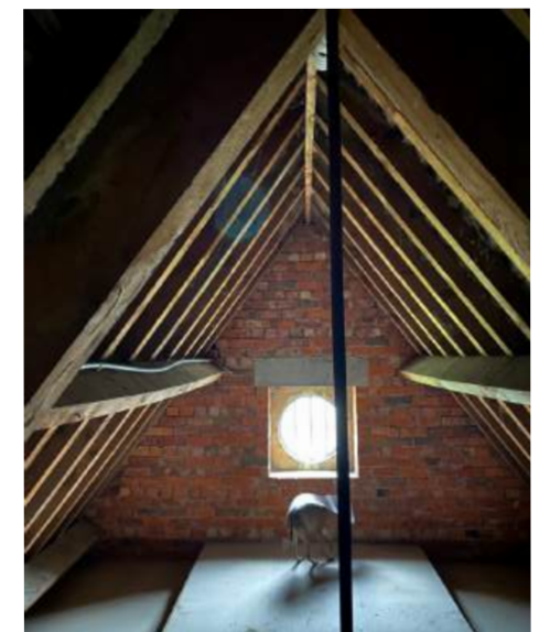
South East Wing - 1919. Roof failures limited to ridges - but the roof is at the end of life.
