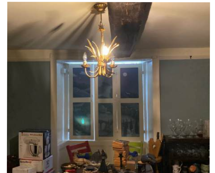
Primary beam mismatched to later opening for sash window
