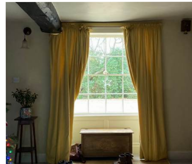
Primary beam mismatched to later opening for sash window
