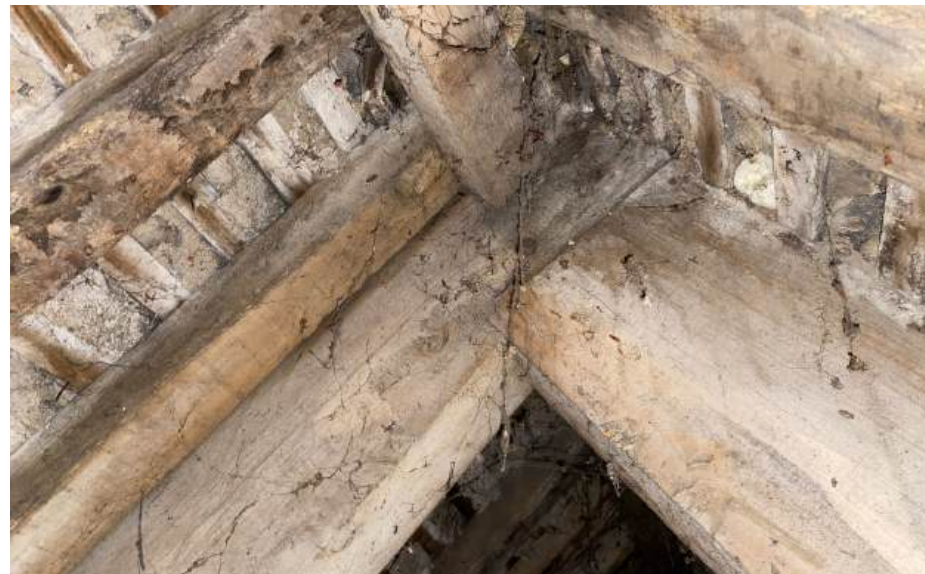
South West (rear) wing roof - Lime torching and iron pegs failing
