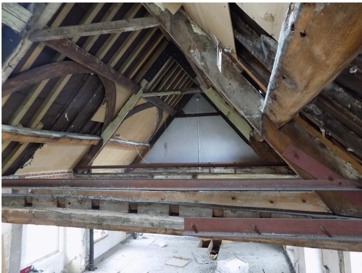
Fig.38: Attic view looking east, showing first tie from east notched for joists along the full length.
