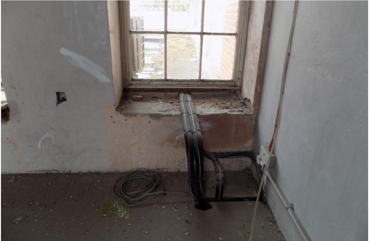
Fig.32: First-floor: Detail of second rear-facing window, showing decayed bottom rail and modern sill.
