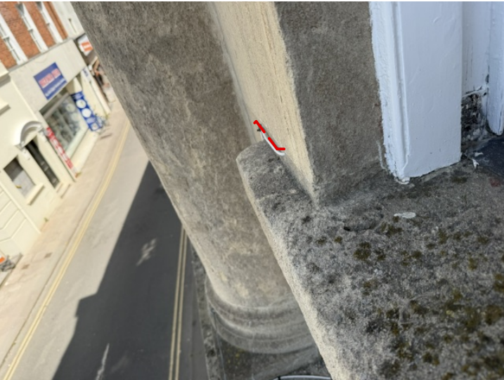
Figure 3: Existing BT electricity cable- external view
