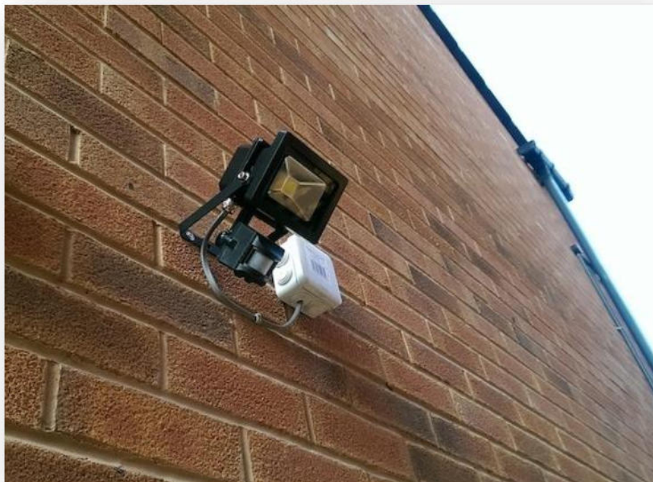
Figure 26b. Directional LED security lighting with sensor
