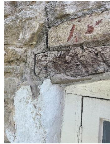
Deteriorated timber lintel to opening
