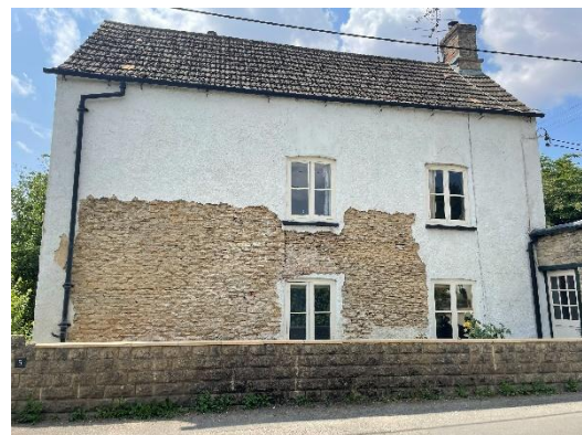
Partial removal of render exposing stone substrate
