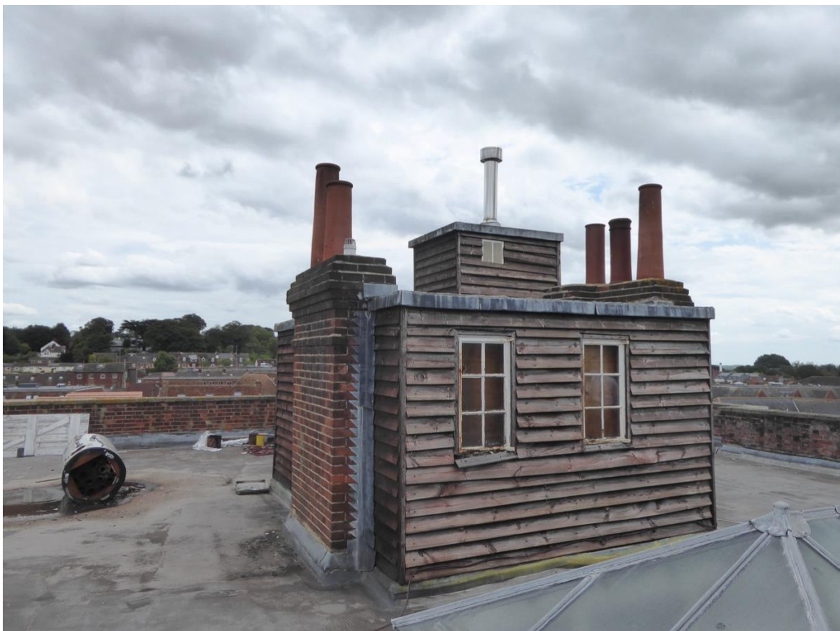
Figure 25: Plant housing set between chimney stacks
