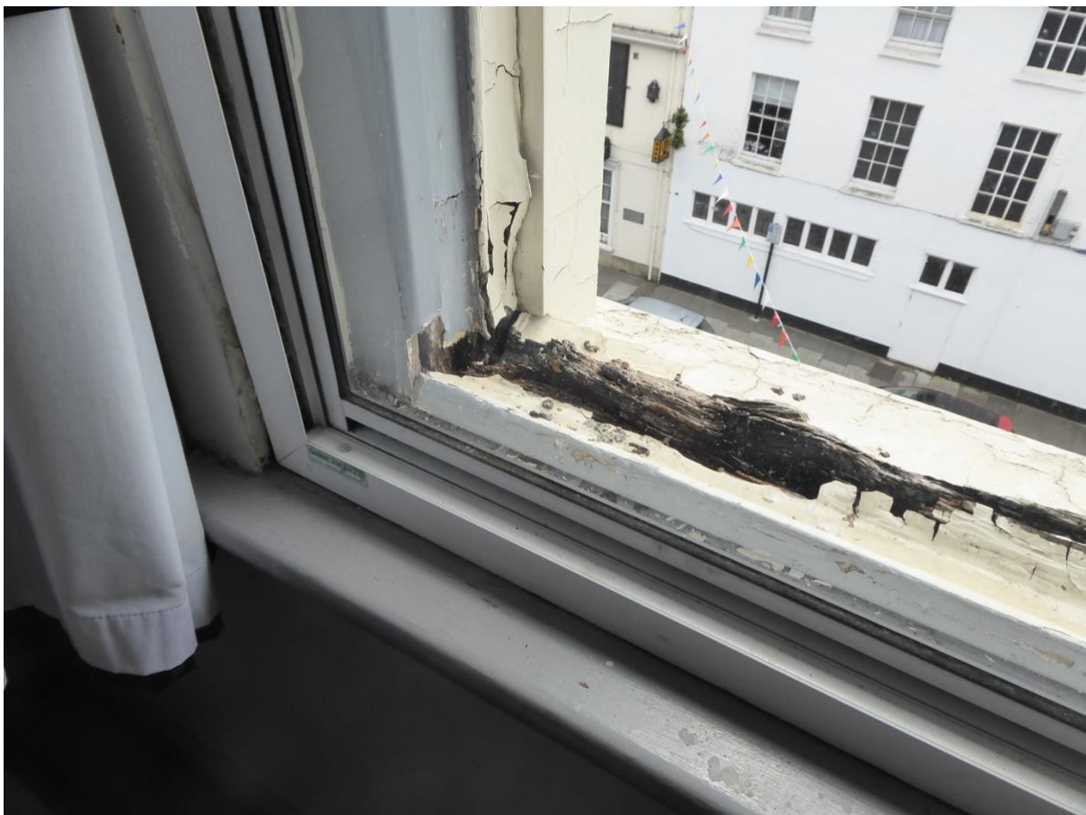
Figure 23: Typical rot pattern of windows associated with many of the sash windows to the front elevation
