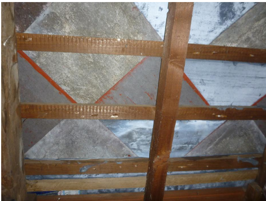
Fig 5: The asbestos roof tiles were unlined (and have since been replaced with slate).
