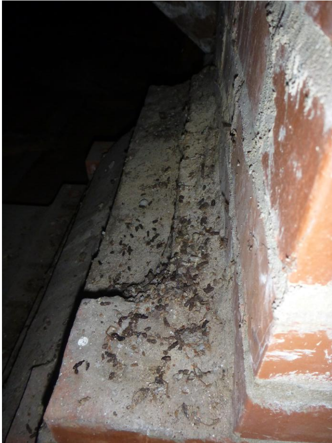
Fig 7: Bat droppings were noted at the base of both chimneys as they pass through the loft space of West Lodge.
