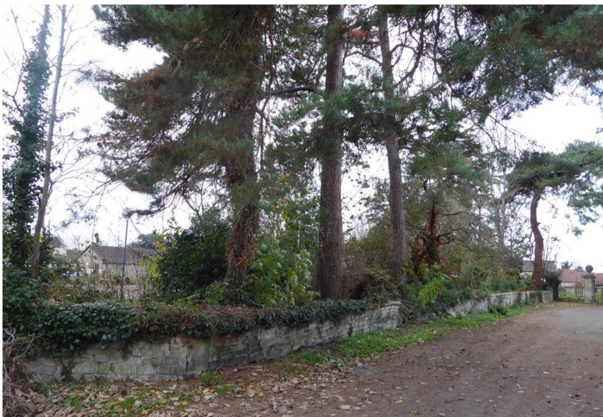
Figure 45: North entrance – low wall attached to gate piers to west of piers
