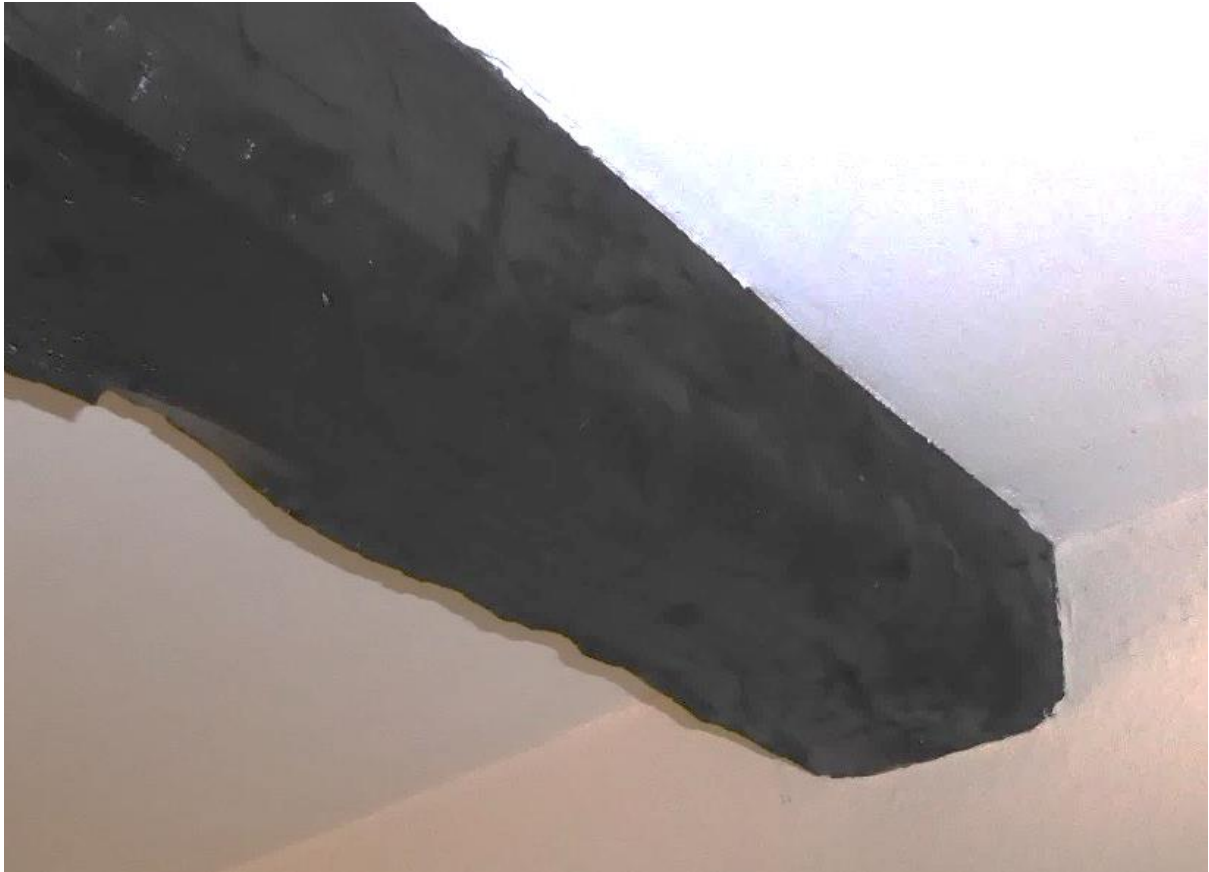
Figure 22: Charred southern end to spine beam in room above kitchen
